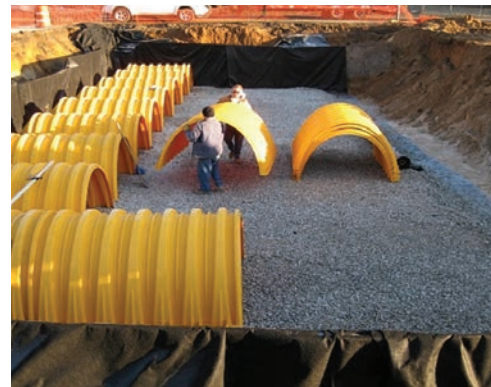
Subsurface Detention Storage
