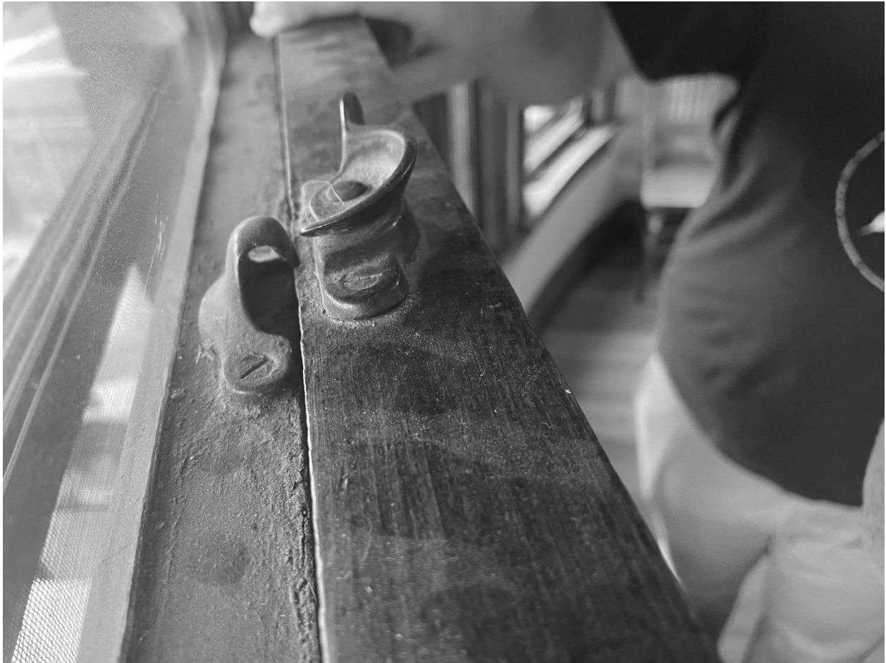
Window #2 – Uneven panes that cannot lock.
