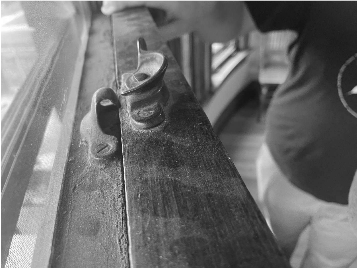
Window #2 – Uneven panes that cannot lock.
