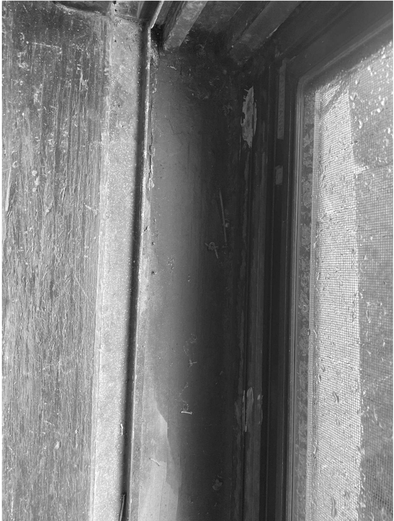
Window #12 – Water Damage
