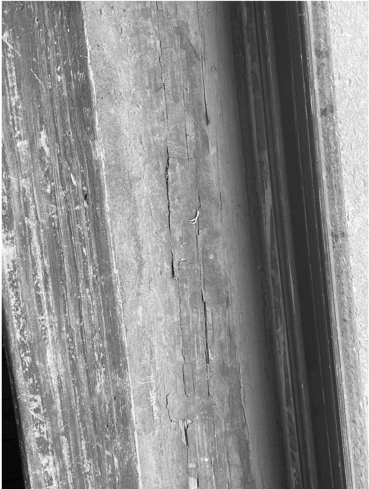
Window #11 – Water Damage
