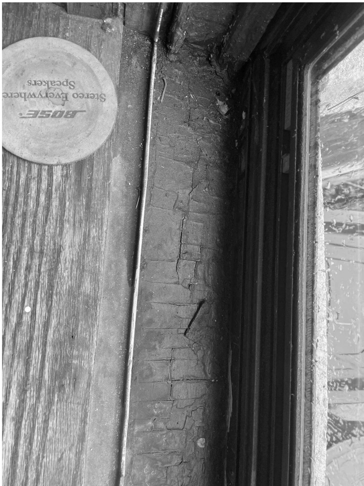
Window #4 – water damage
