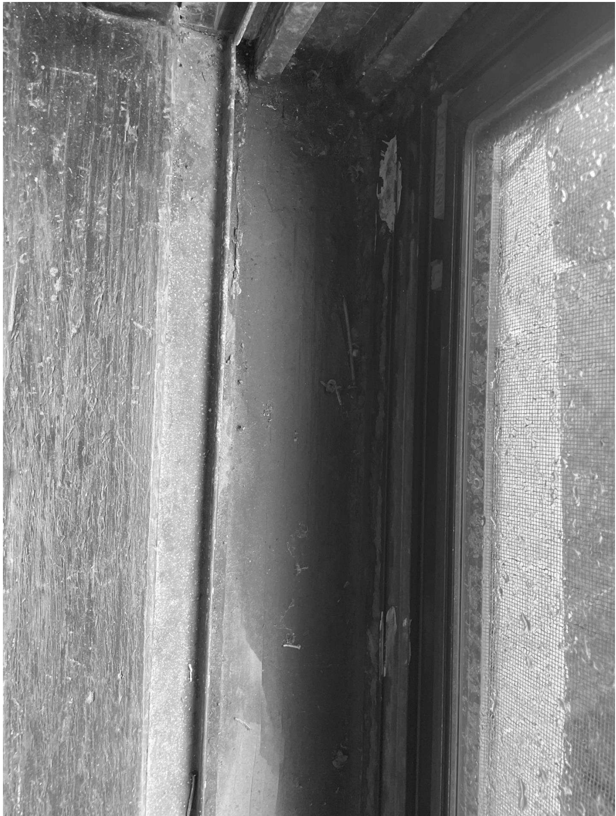
Window #12 – Water Damage
