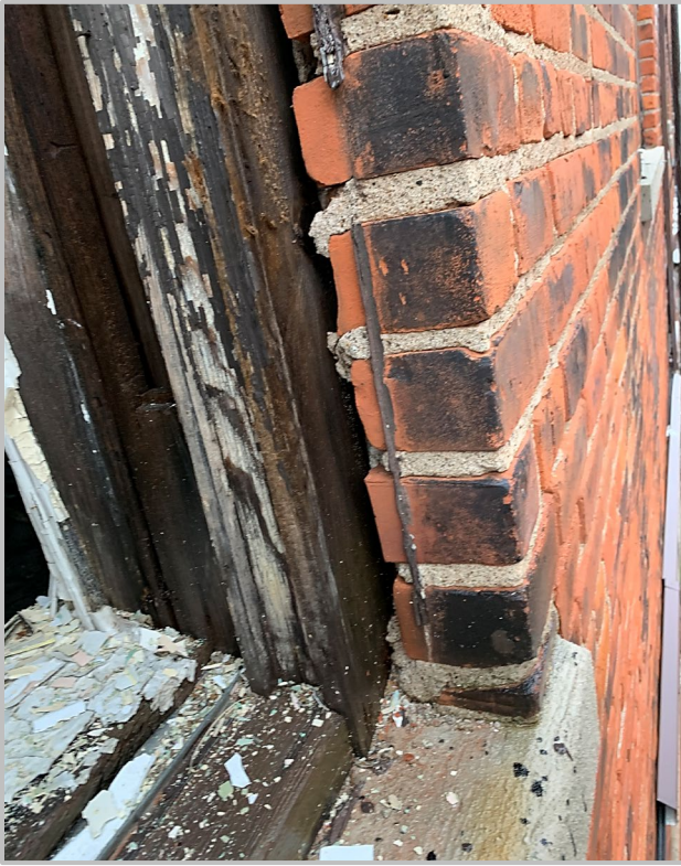
Photo 5: Exterior View of Sill, Jamb, and Frame with Missing Brickmould (a common condition)
