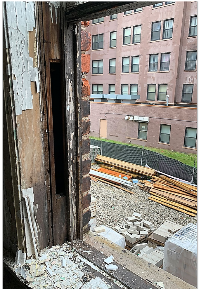
Photo 6: Interior View of the Window - Jamb, Sill, and the Missing Sash
