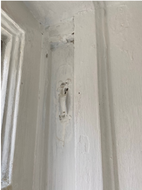
Operating hardware missing or inoperable
