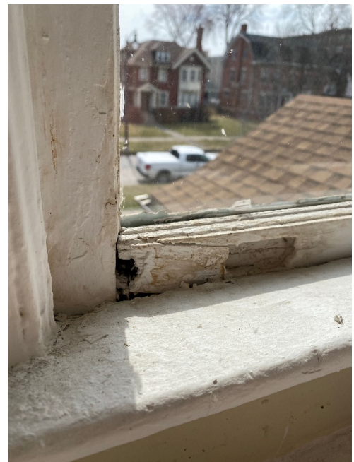
Rot at window sashes
