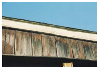
Not back primed. Weathered wood and mold
