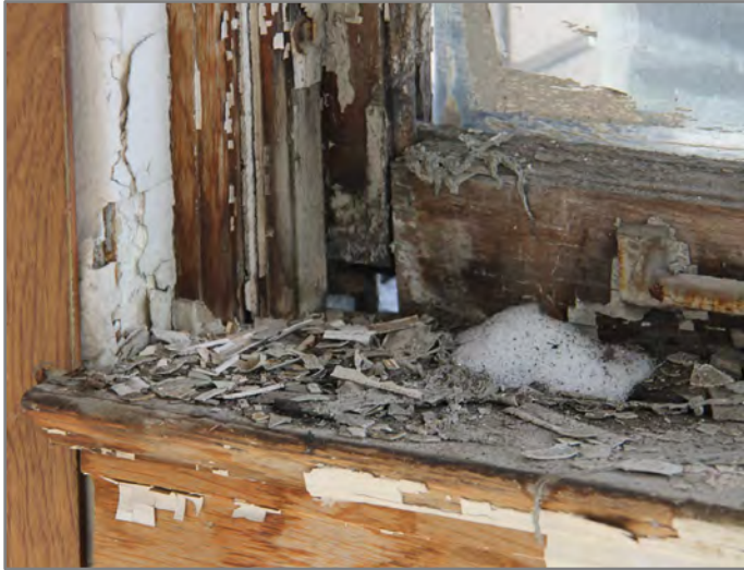
Interior View of Wood Double-Hung: Deteriorating Side Rail and Bottom Rail
