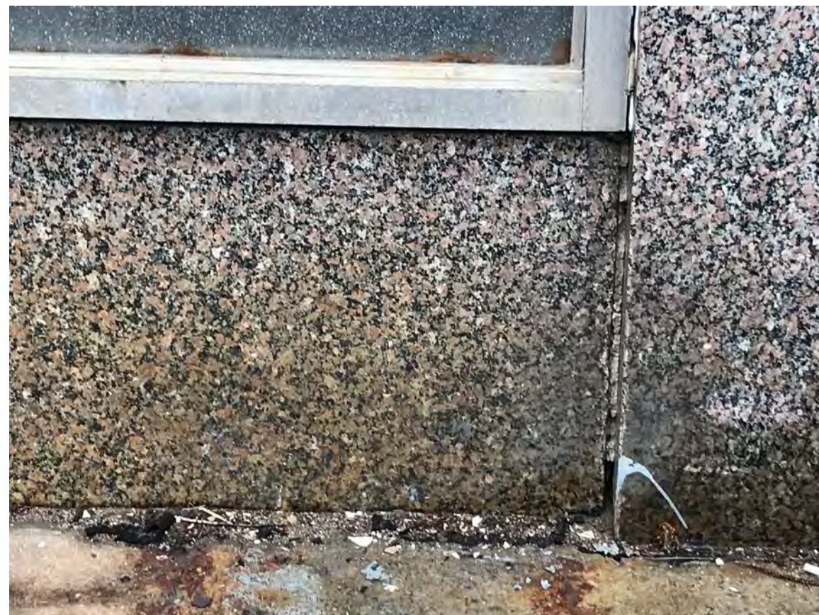
EXISTING CONDITION OF GRANITE, TYPICAL BELOW STOREFRONT SILL
