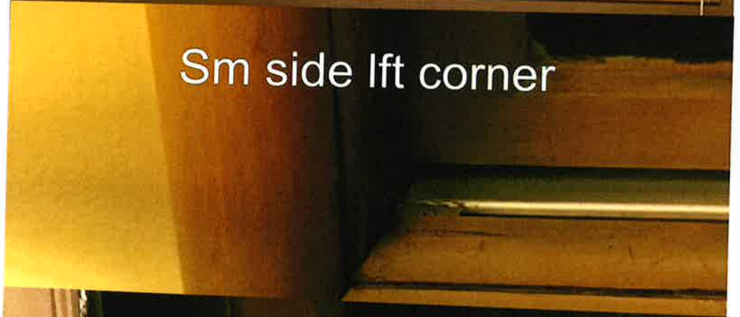
Sm side gap in pane
