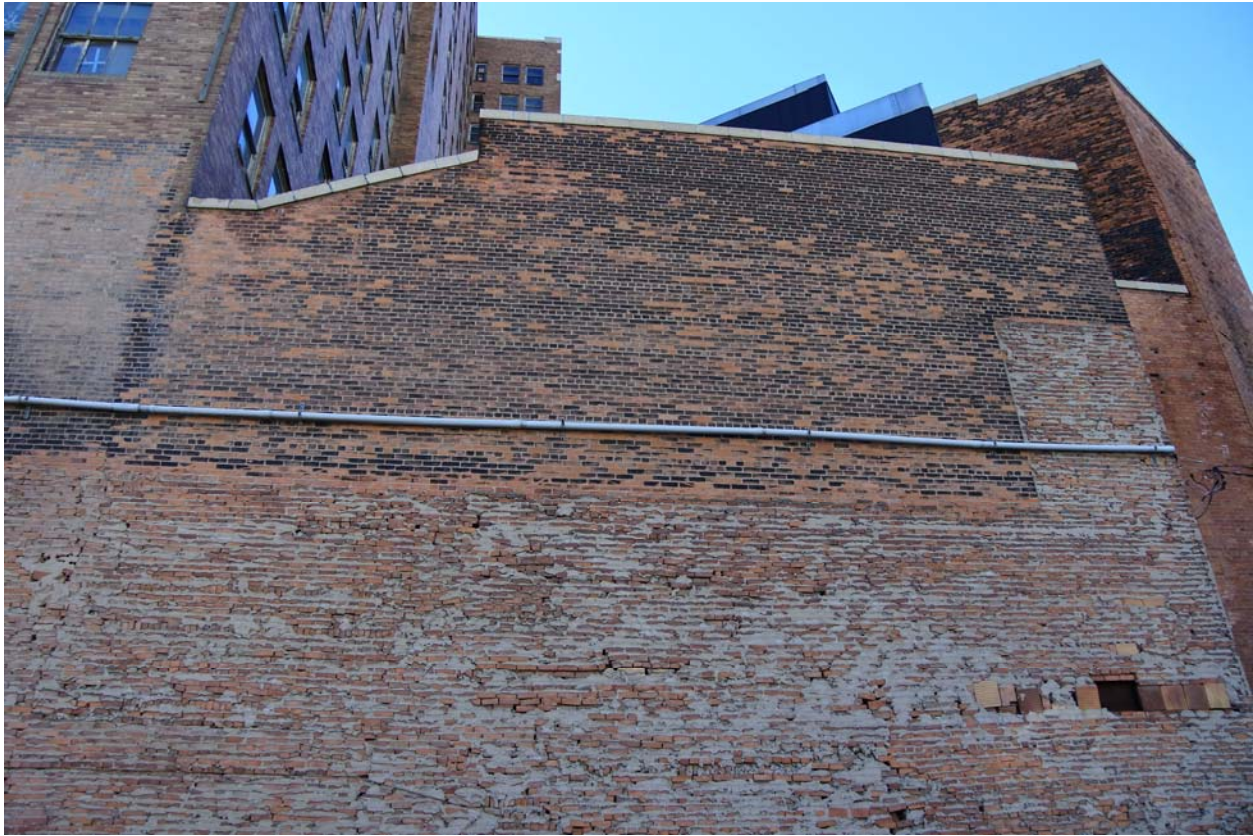
Image #28 – Area of rubble brickwork on the north elevation that was not originally an exterior wall surface. Most if not all of the north wall will either need to be parged and covered with another material, or rebuilt as a brick veneer with masonry back-up wythe.
