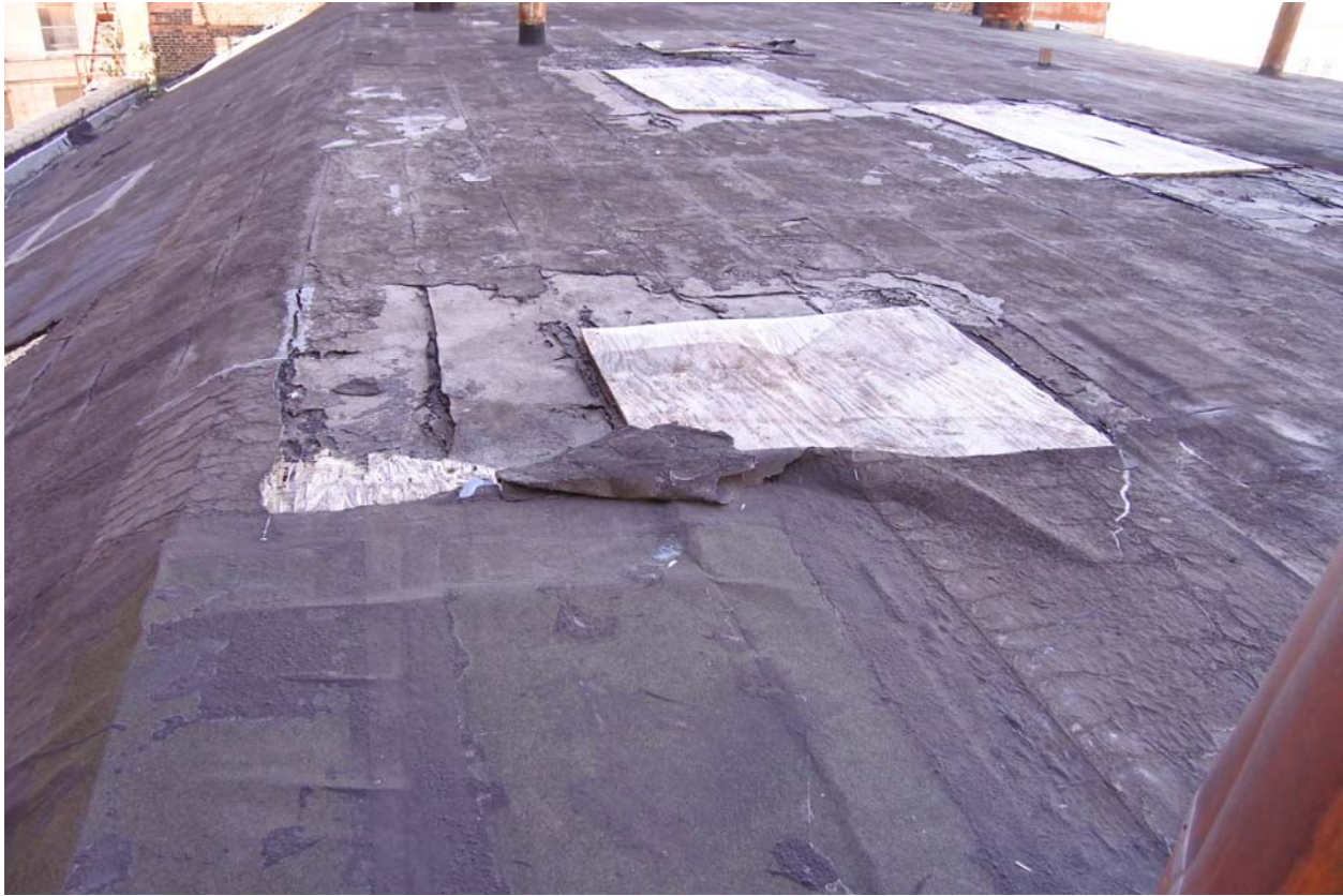
Image #23 – Roof has several plywood panels and poorly constructed patched areas.
