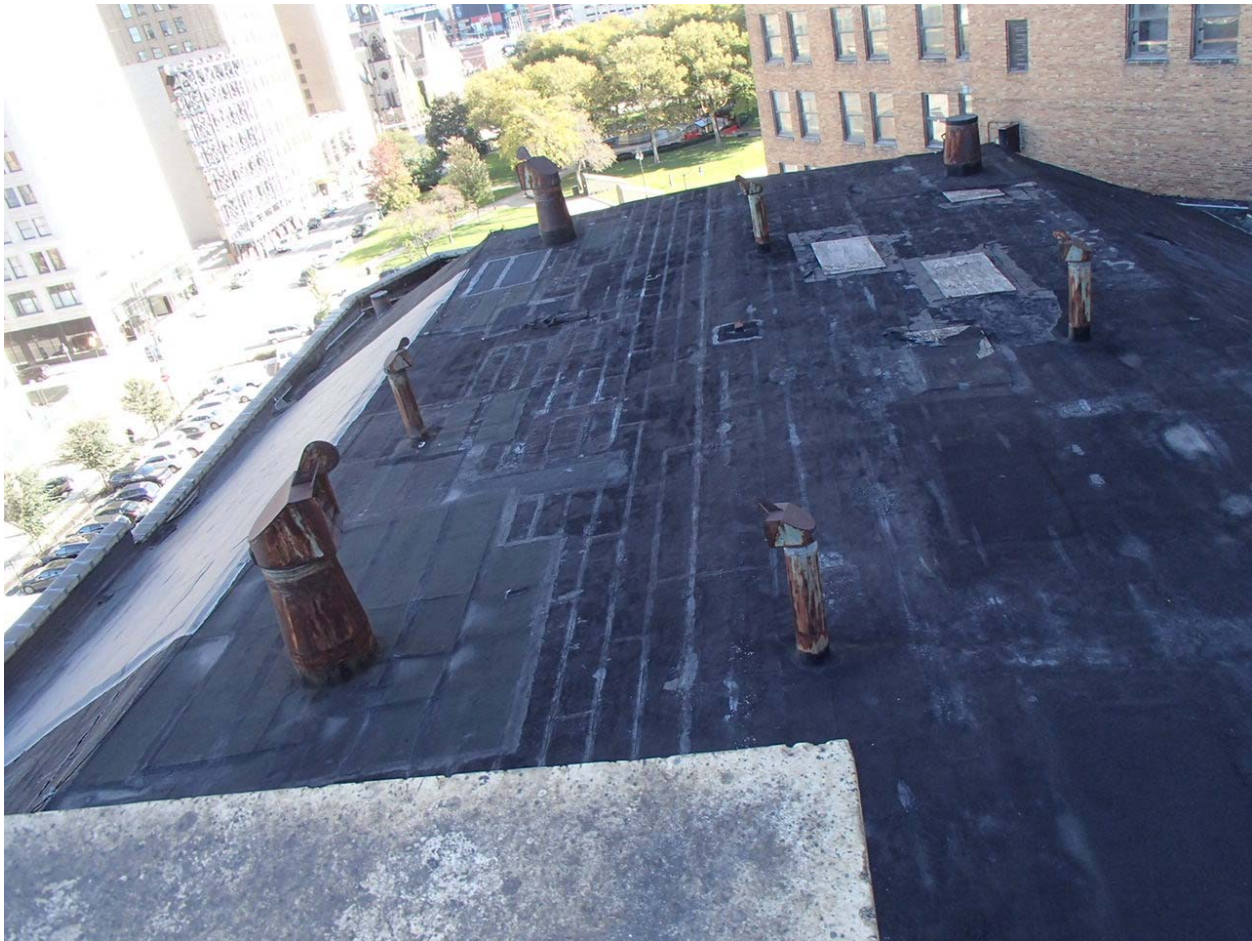
Image #13 – Main roof above theater seating area viewed from high roof above the fly loft. Gutter formed by roofing flashed to very short parapet along exterior wall has leaked water into exterior brick bearing wall below. With no railing and such a short parapet, the access to clean the drains and maintain the flashings is dangerous. The failed gutter and parapet coping and flashing has resulted in significant damage to the exterior brick wall below. We estimate 50% of the brick on the west façade will require repair and/or replacement as a result of this condition.
