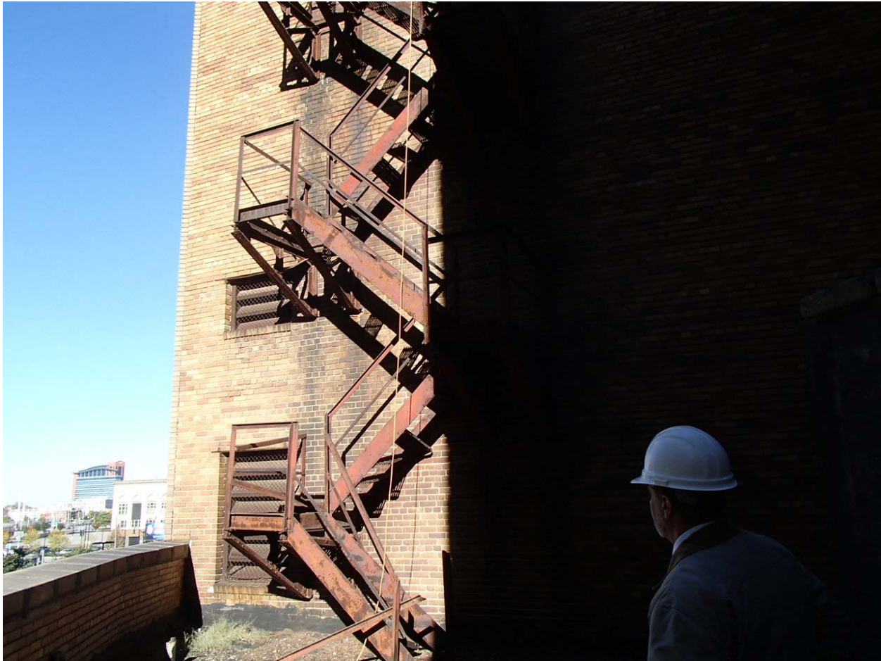
Image #9 – Exterior fire escape is unsafe as it is missing several treads.
