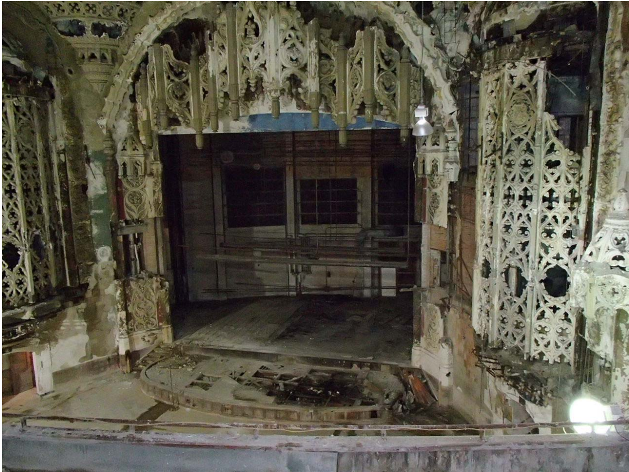
Image #11 – Portion of stage with curved front edge is a vertically operable section of floor with wood floor deck and framing spanning between steel beams. The wood framing has severely deteriorated due to water intrusion.
