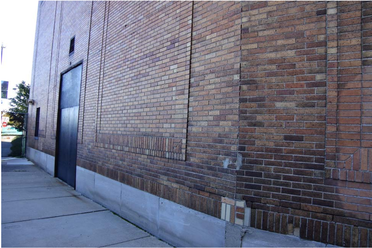
Image #25 – The exterior brick on the lower portion of the Clifford Street side appears to be in good condition with minor repairs required at the corners however the brick near the top of this wall is pulling away from the back-up wythe and must be re-anchored. The sidewalk here should have a protective roofed scaffold constructed until repairs can be made.
