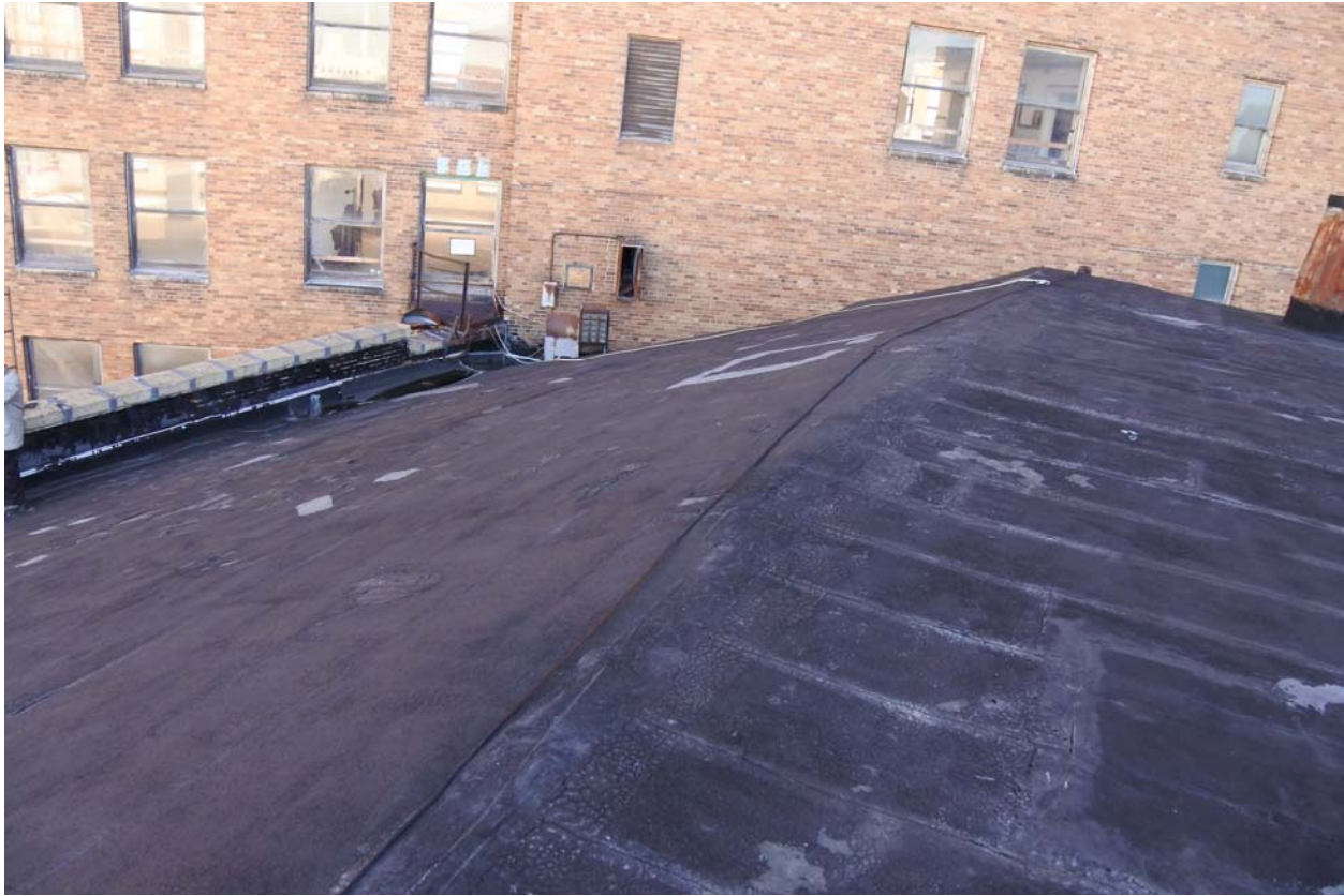
Image #21 – Typical view of main “egg shaped” roof. Structure below is steel trusses and purlins supporting a gypsum plank roof deck. Photos and written report by others done in 2007 indicate the gypsum deck is heavily water damaged, and sagging, and must be completely replaced.
