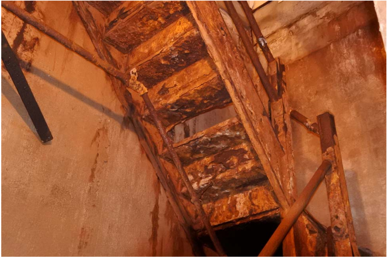
Image #16 – Rusted stairs to lower level.
