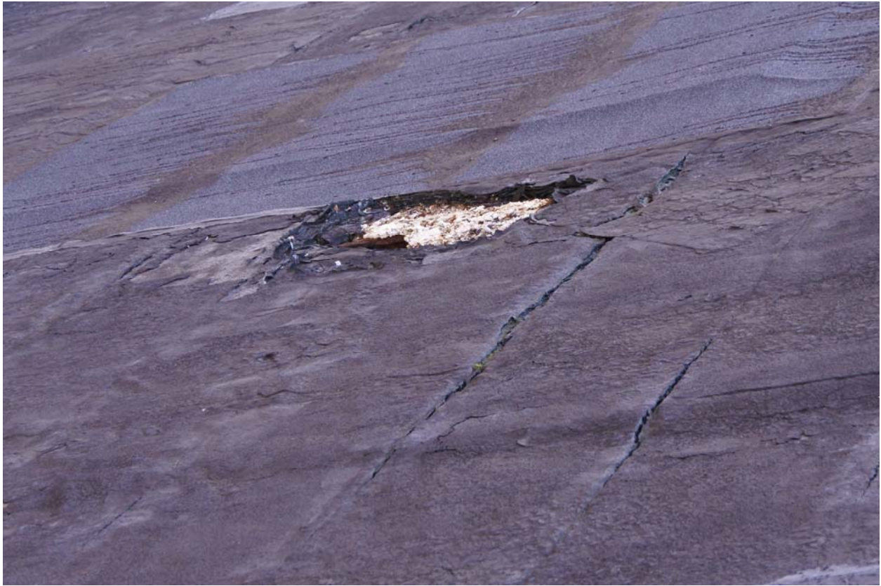
Image #22 – Roof damage
