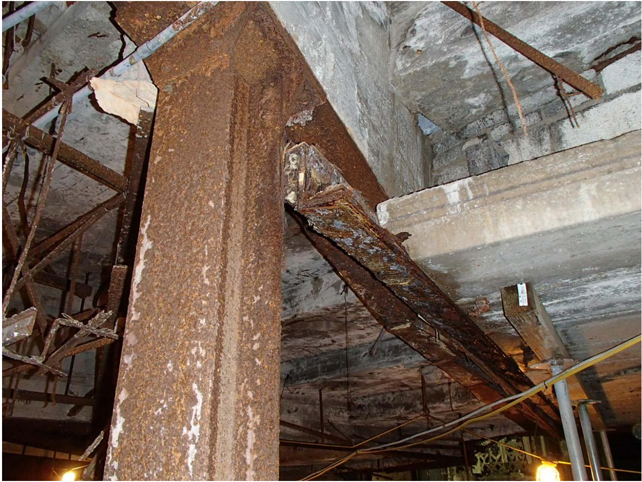
Image #1 - Rusted steel angle supporting concrete balcony floor slab. This corroded steel would need to be completely replaced.
