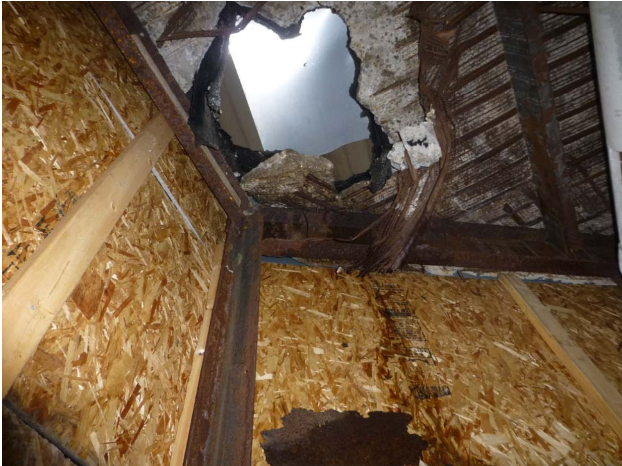
Image #36 – Photos sent by Fred Beal that were taken in June 2013 showing condition of underside of main roof above the seating area.
