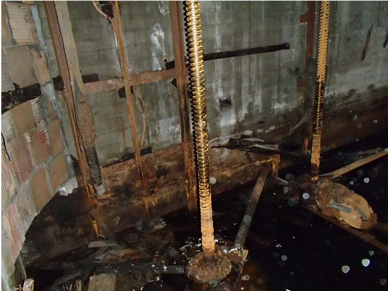
Image #5 – Screw jack mechanism for moveable stage floor. Water intrusion into the orchestra pit will need to be investigated further and mitigated.
