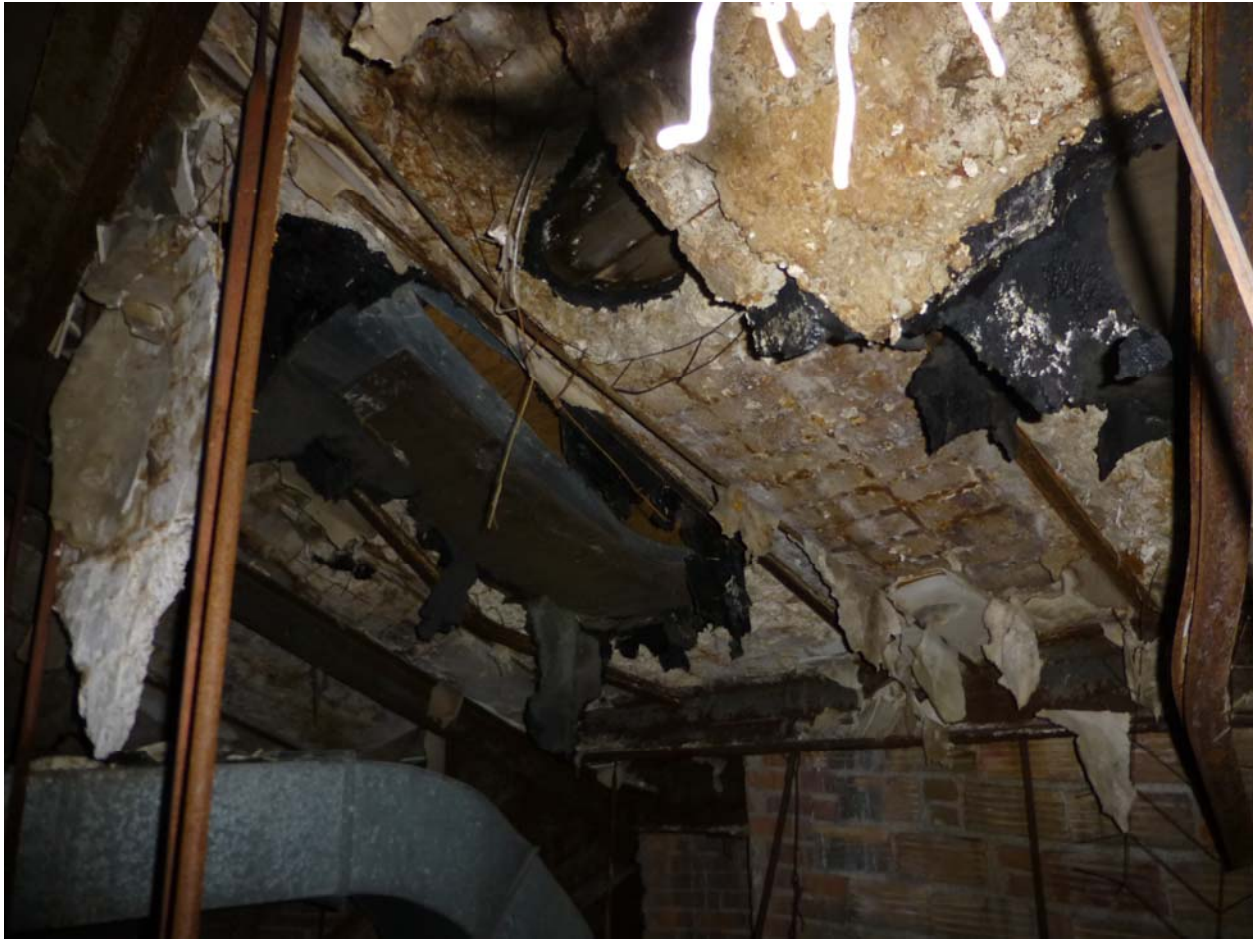
Image #38 - Photos sent by Fred Beal that were taken in June 2013 showing condition of underside of main roof above the seating area.
