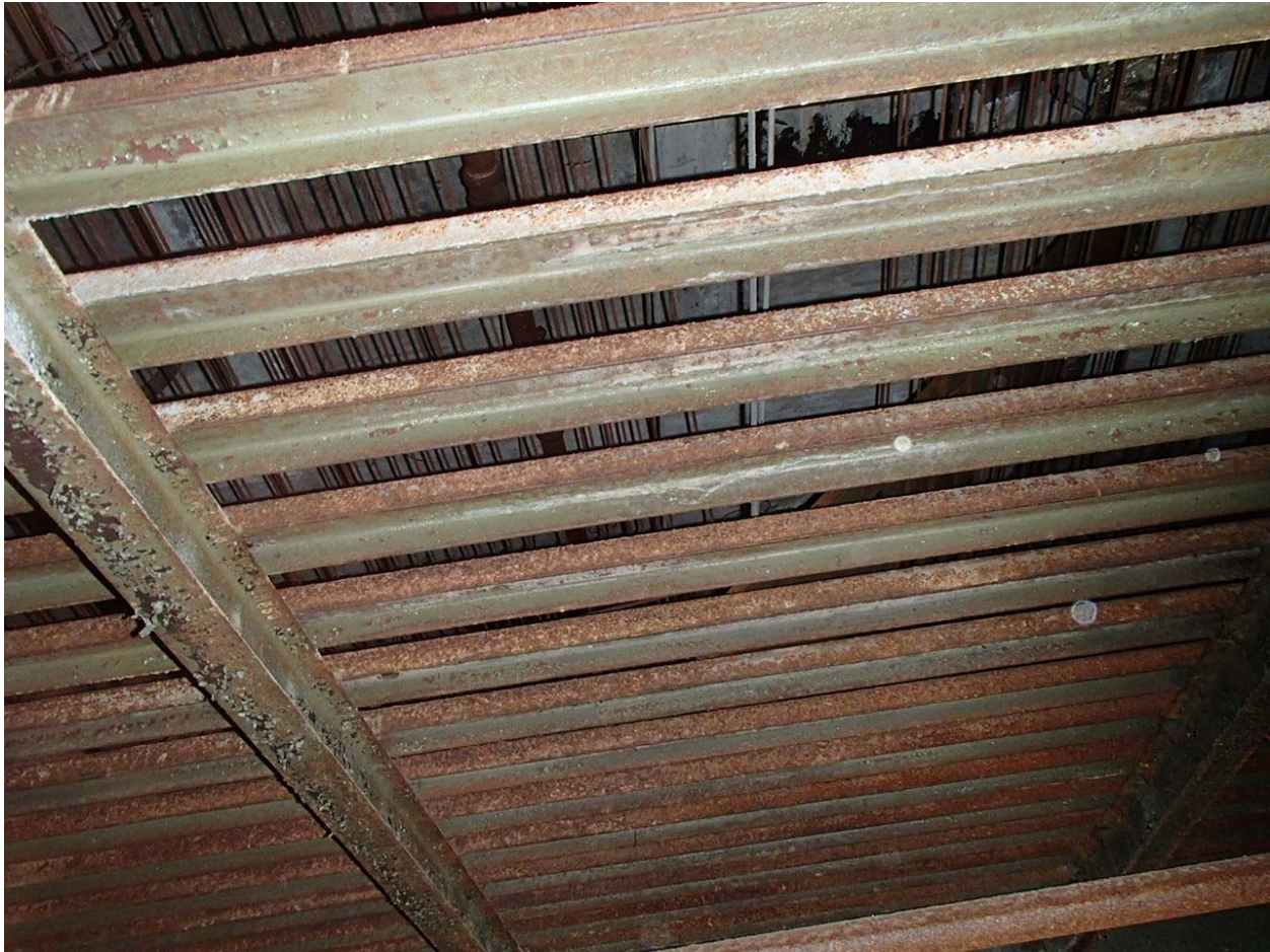
Image #7 – Grid iron floor above the stage has surface rust. This area is below the flat roof above the fly tower, which has been kept relatively water tight. The remainder of the theater space below the “egg shaped” roof was not kept water tight and has much more severe deterioration of the structure below.
