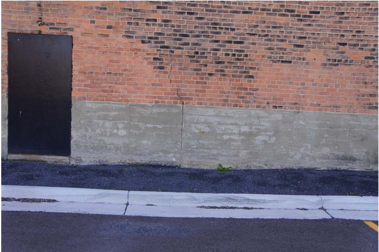
Image #30 – Cracks in exterior brick wall above joint in concrete foundation wall. The bricks above the concrete should be re-worked so that a control joint in the brick corresponds to the joints in the foundation wall.
