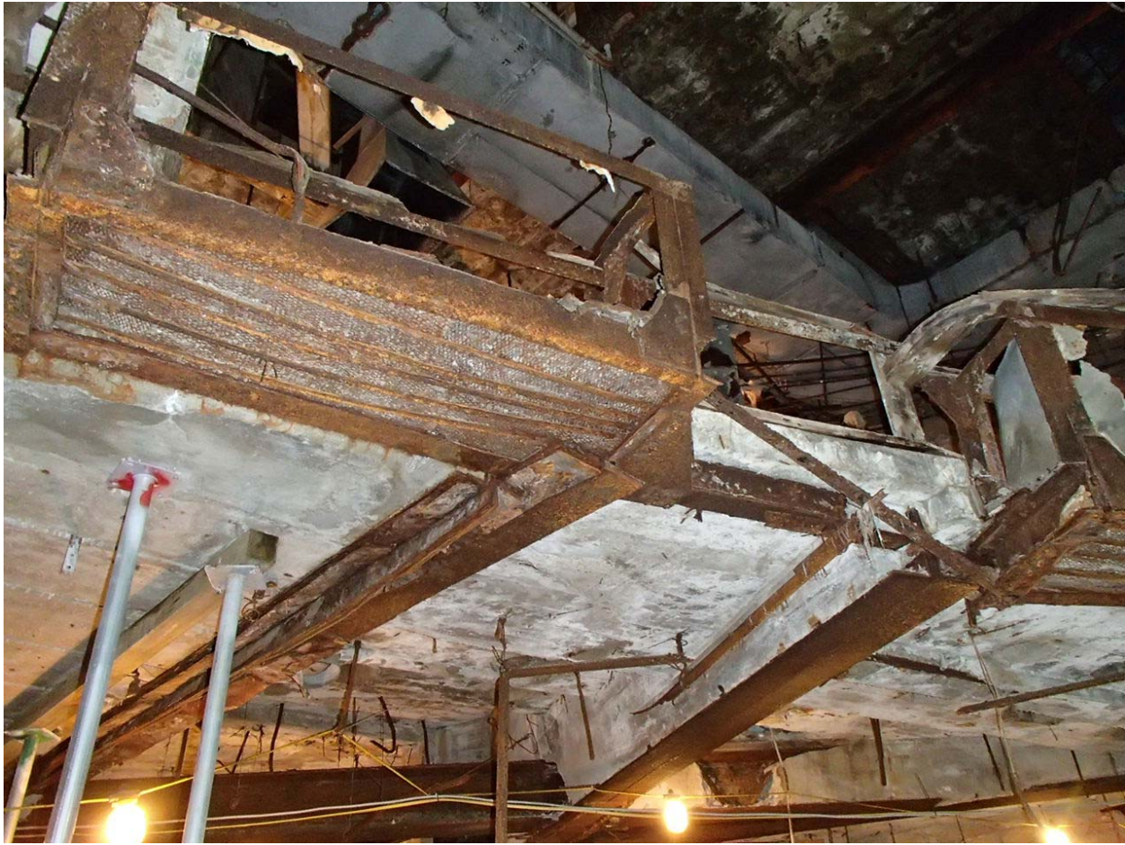
Image #3 – Rusted steel support at front edge of balcony. Much of this corroded steel would need to be completely replaced.
