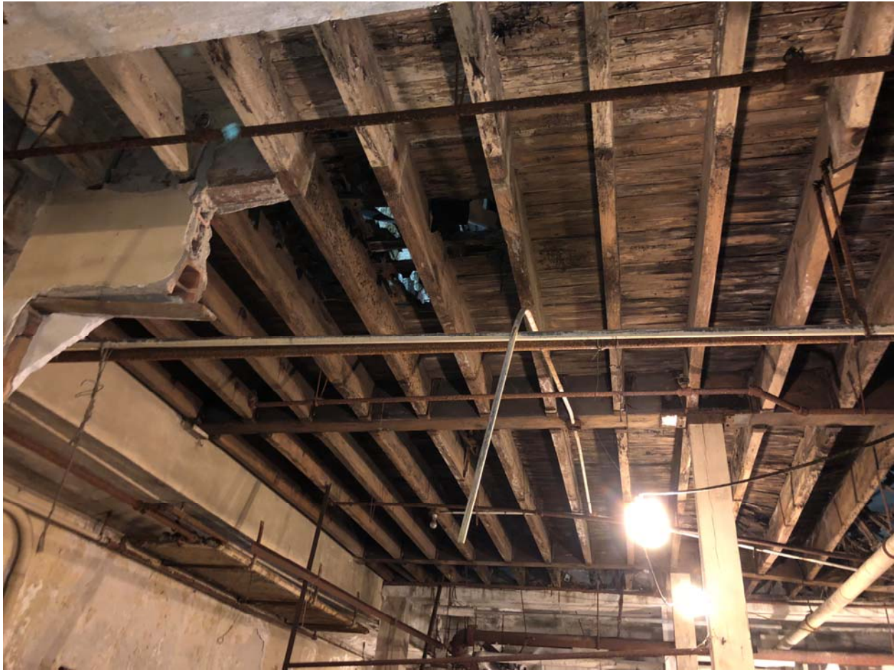
Image #34 – Underside of wood framed area of stage floor. There is much water damage to this area due to roof leakage. All of this wood framed floor must be removed and replaced.
