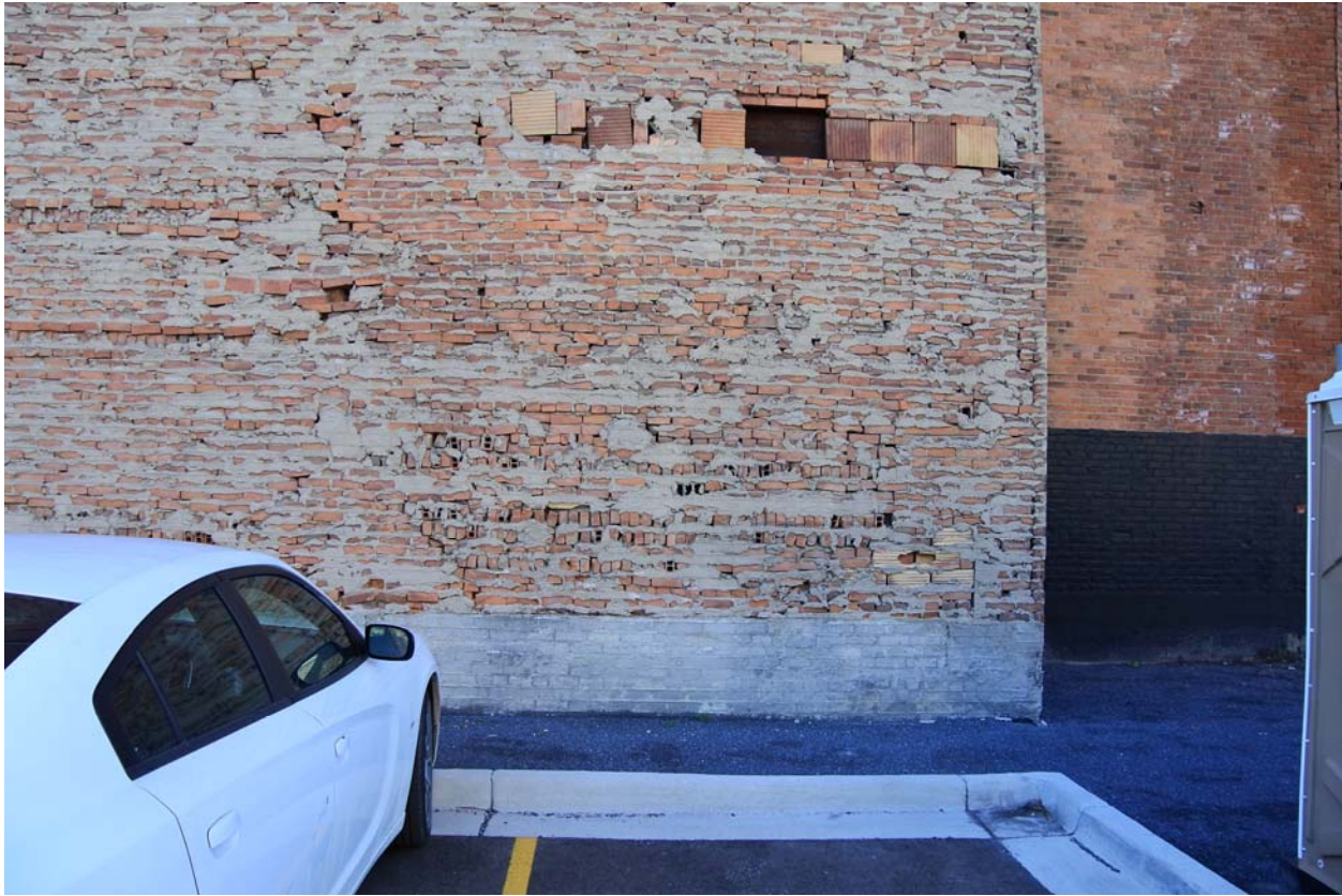
Image #29 – Area of rubble brickwork on north facade that was not originally an exterior wall surface. Most if not all of the north wall will either need to be parged and covered with another material, or rebuilt as a brick veneer with masonry back-up wythe.
