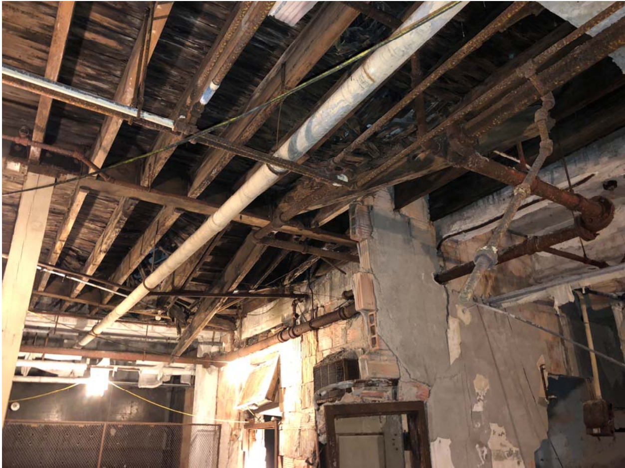
Image #35 - Underside of wood framed area of stage floor. There is much water damage to this area due to roof leakage. All of this wood framed floor must be removed and replaced.
