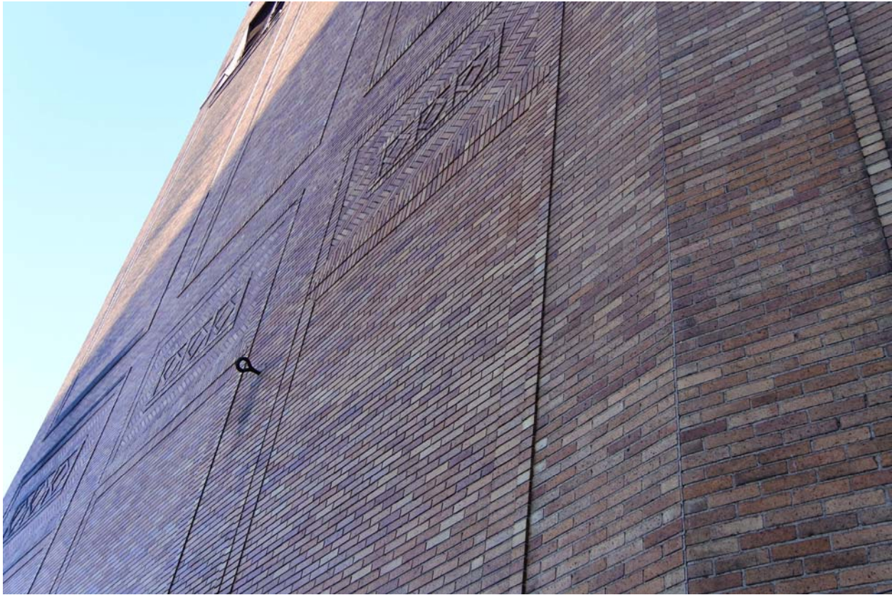
Image #24 – Photo of the lower portion of the exterior brick on Clifford Street ( south elevation ) is in good condition however the brick near the top of this wall is pulling away from the back-up wythe and must be re-anchored. The sidewalk here should have a protective roofed scaffold constructed until repairs can be made.
