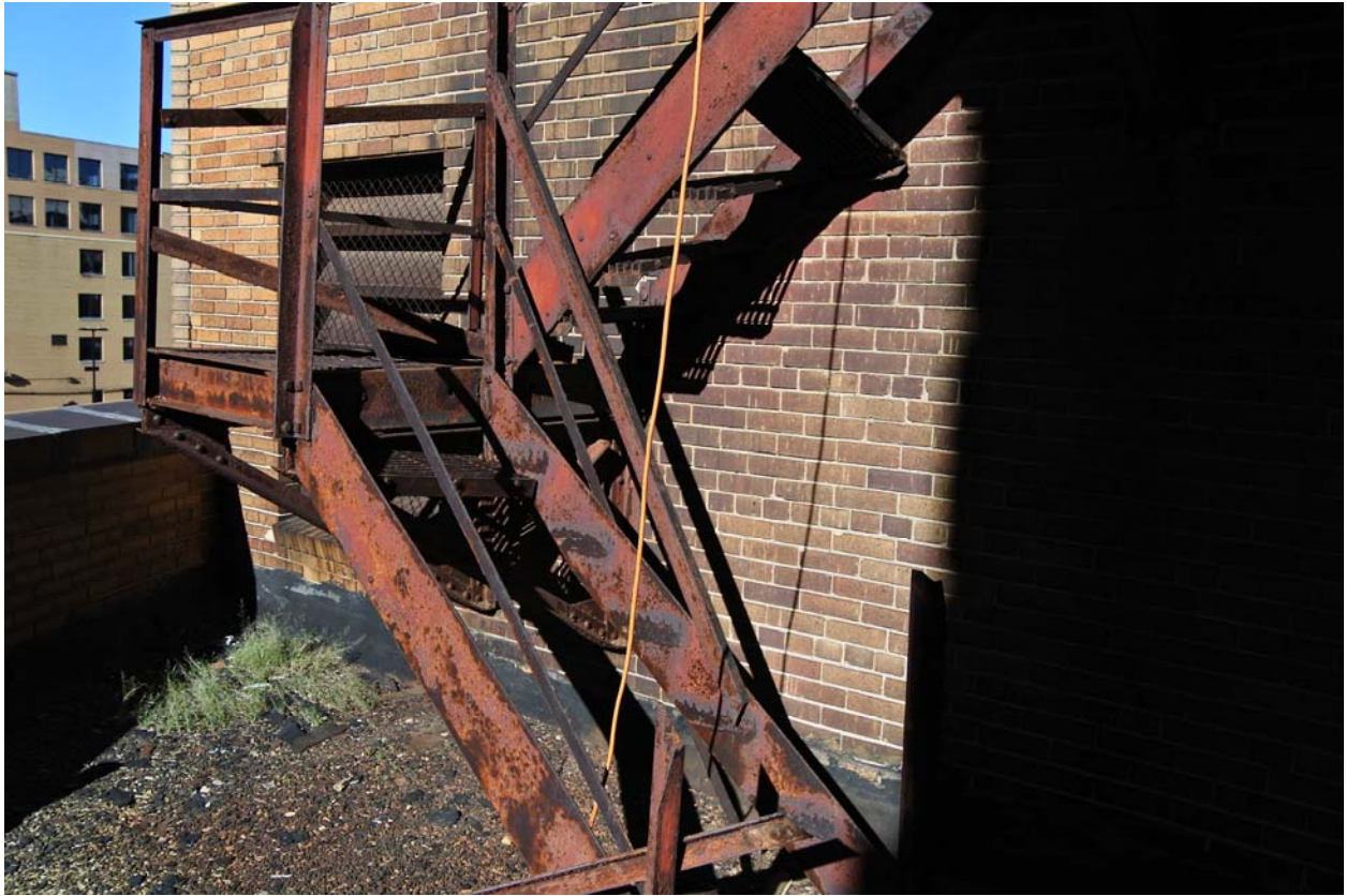
Image #18 – Rusted fire escape with missing treads.
