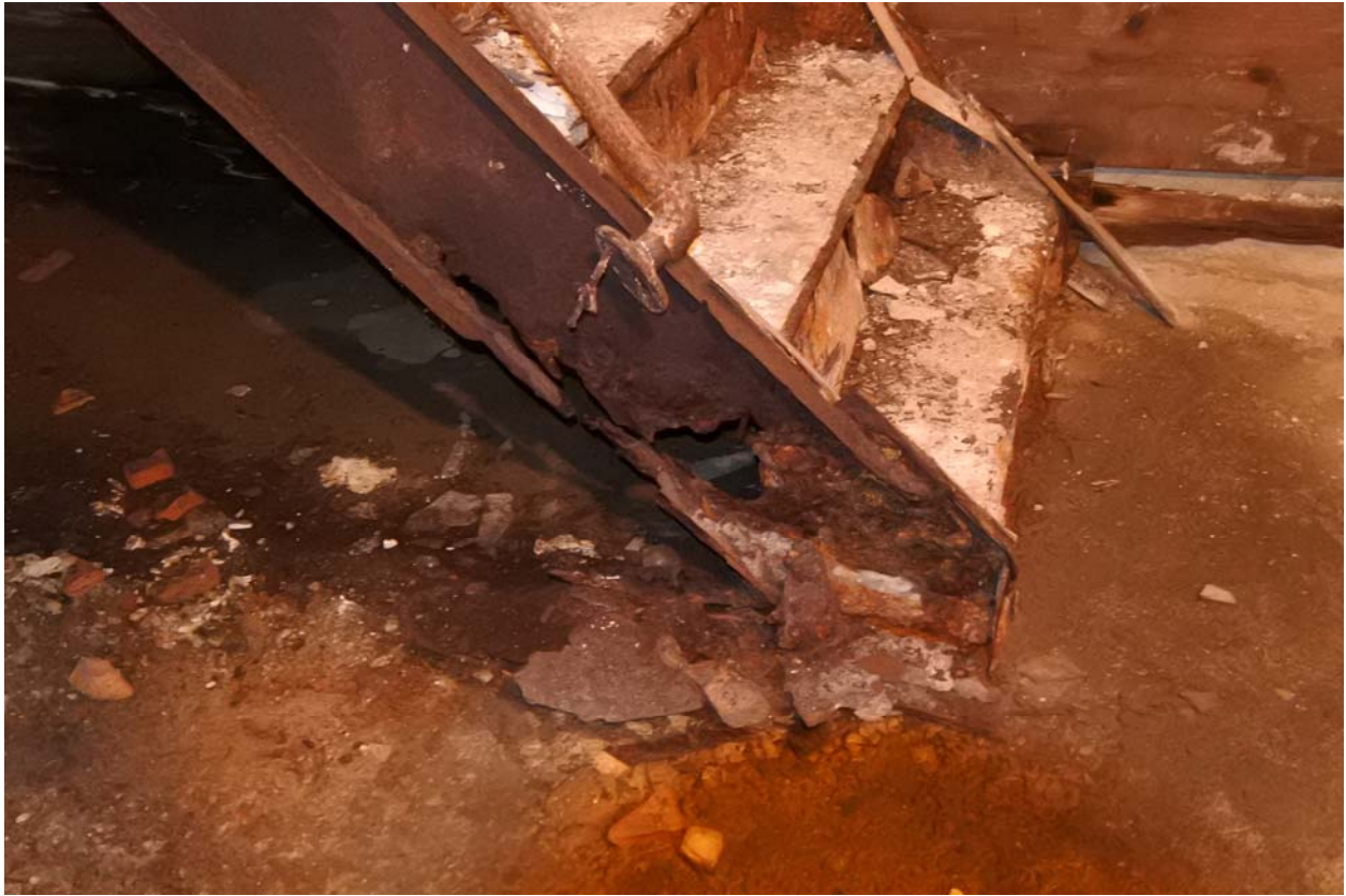
Image #17 – Rusted stairs.
