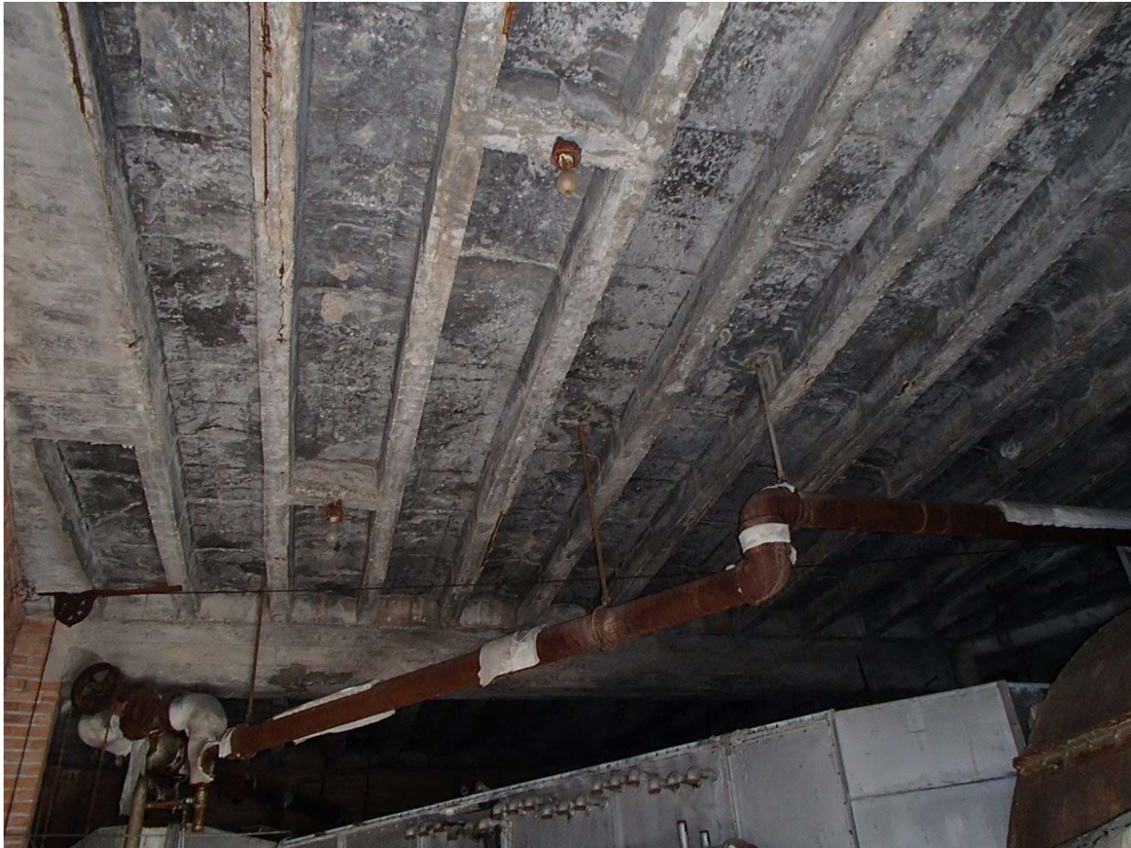
Image #14 – Underside of flat roof structure of fly tower - note there is some spalled concrete at rusted rebar locations.
