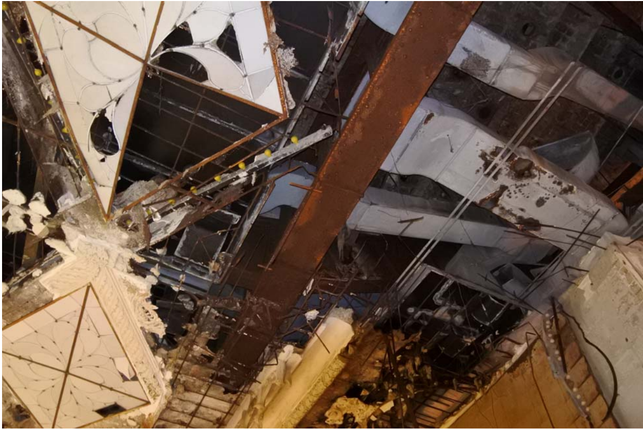
Image #19 – Underside of balcony has heavy plate girder supporting built-up steel “raker” beams that appear to have only surface rust where they are exposed. Less than half of the balcony framing could be observed due to some ceiling finishes still being in place.
