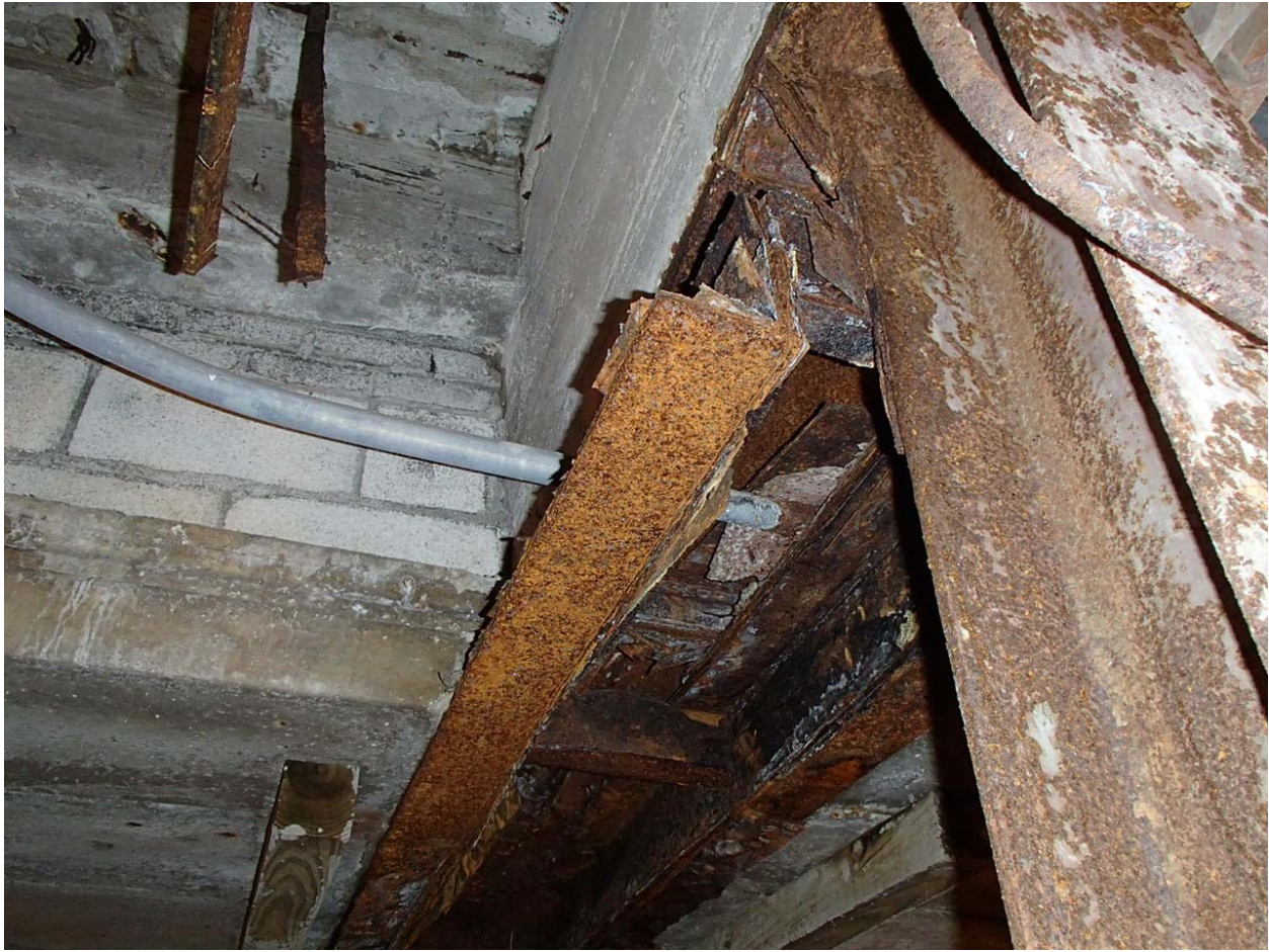
Image #2 - Rusted steel angle supporting concrete balcony floor slab. This corroded steel would need to be completely replaced.
