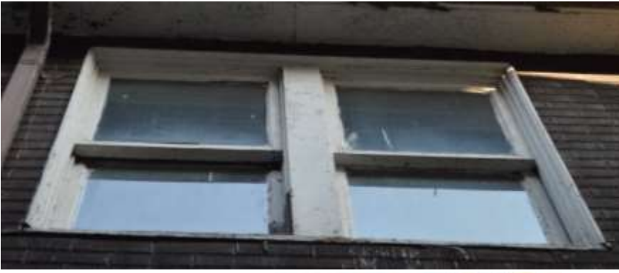
16 – Rotted sill and frame, bottom sash rotted, sash warped
