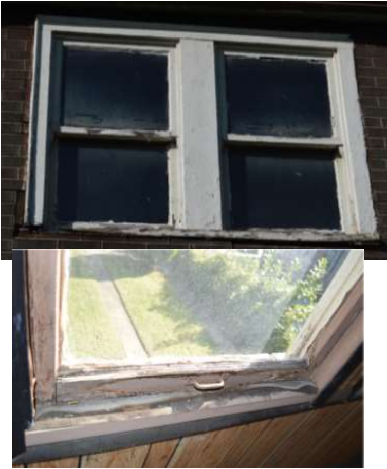
20 – Rotted sills and sash
