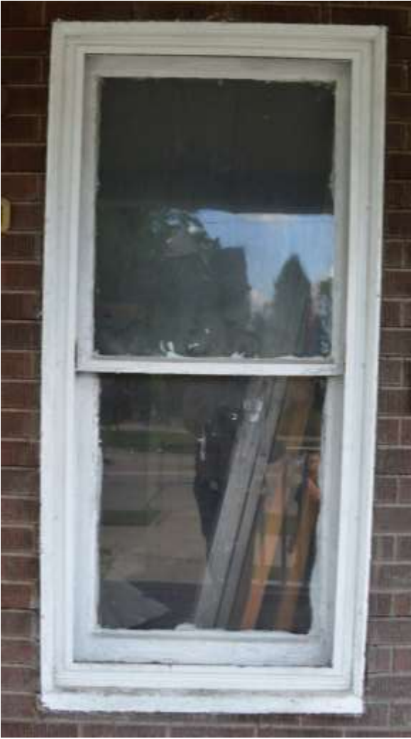
4 - Frame and bottom rails of sash are rotted
