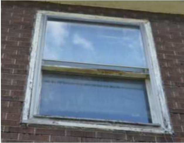
14 – upper sash rail eaten away, rotted sill
