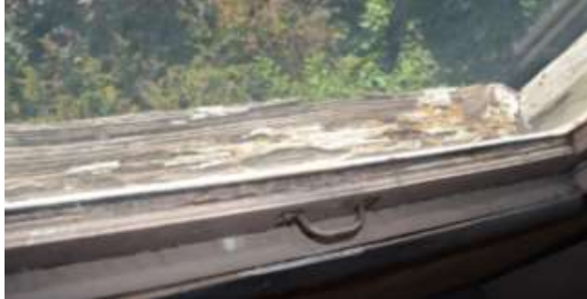
19 – Rotted sill and sash
