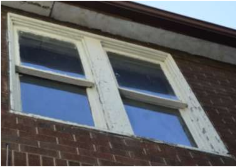
22 – interior taped together, bottom rails rotted
