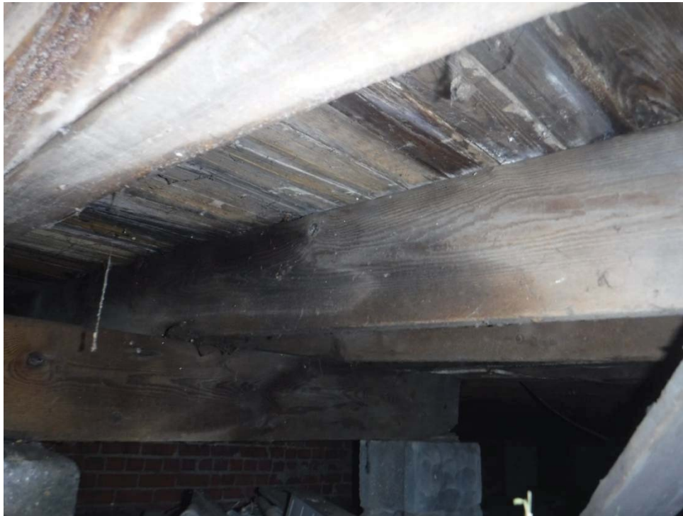
Photo 38: Crawl space floor joist at the rear
