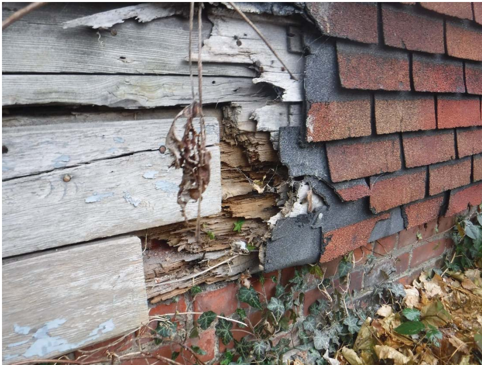
Photo 36: North-east corner with damaged wood siding.
