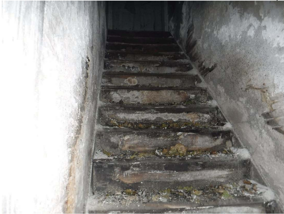
Photo 31: Stairs up to 2 nd floor. Stringers and steps are soft.
