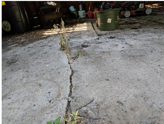
FIGURE 4 – SLAB CRACK ACROSS THE LENGTH OF THE SLAB
