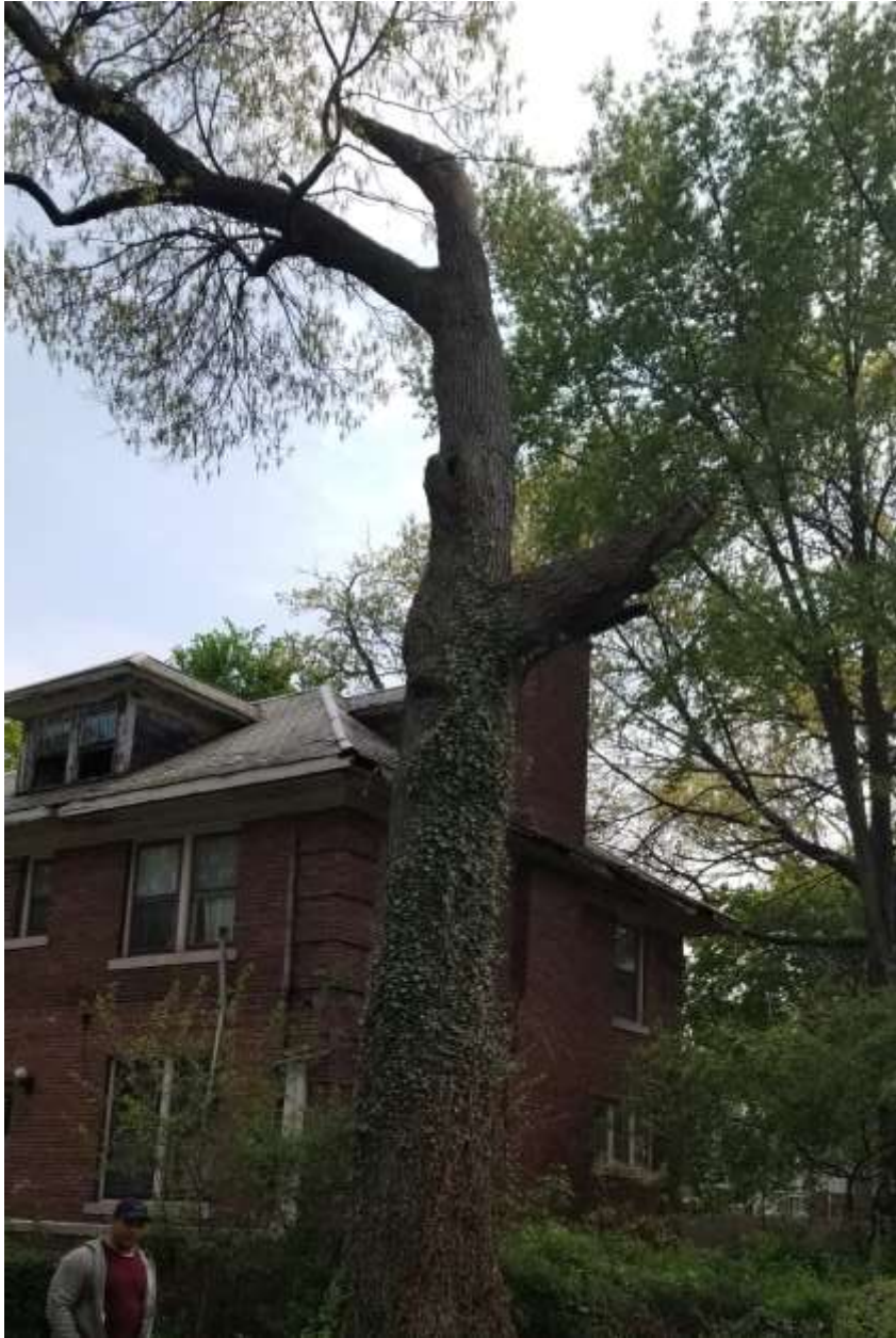
Half cut and overhanging the roof, which is potential for roof damage, unattractive and detracts from curb appeal
