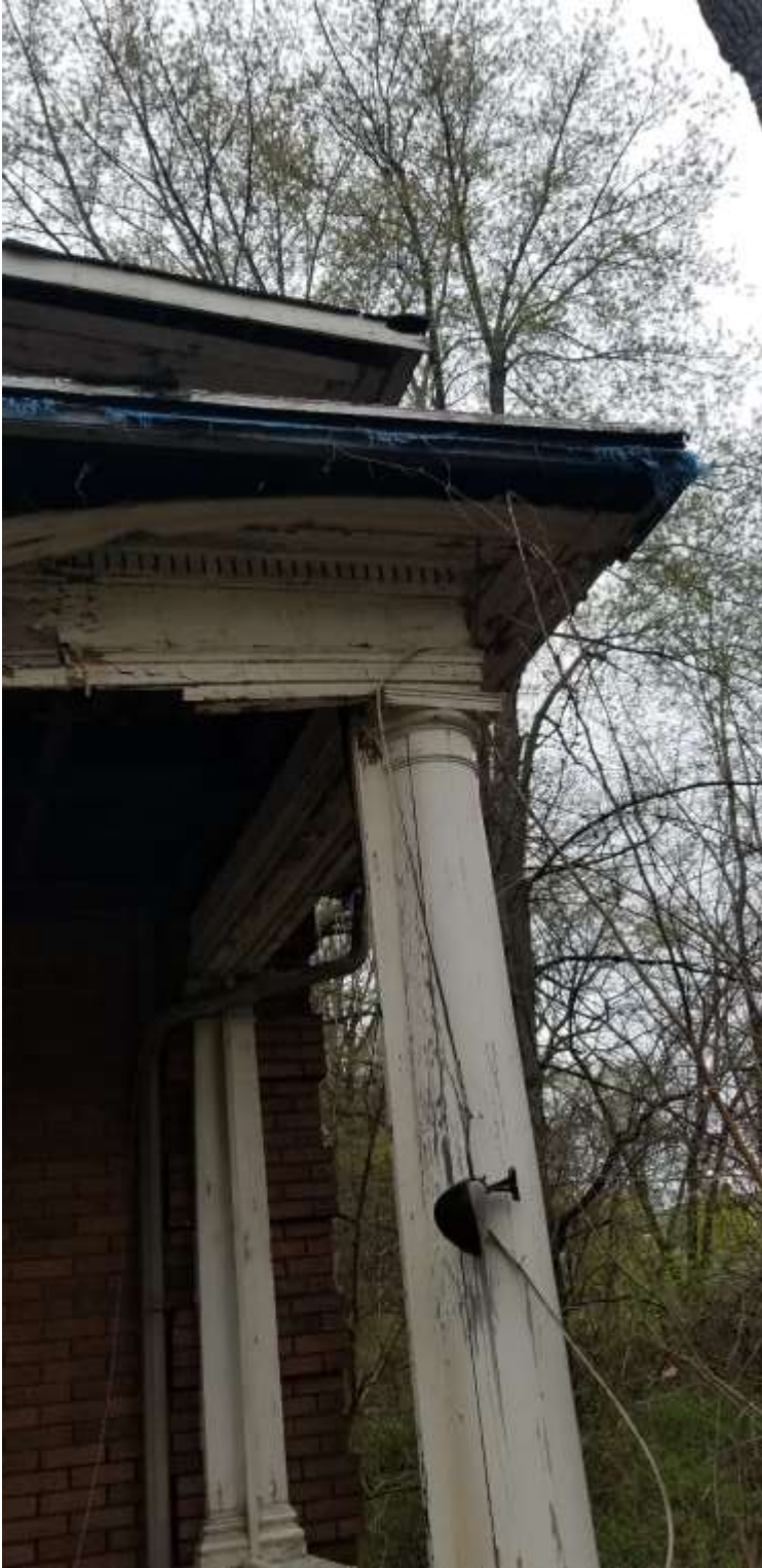
Structural porch members split and water logged and disintegrated
