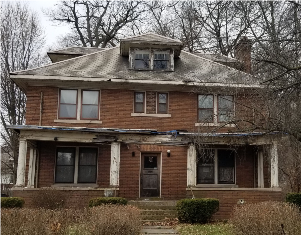
3457 Iroquois, porch prior to unapproved removal
