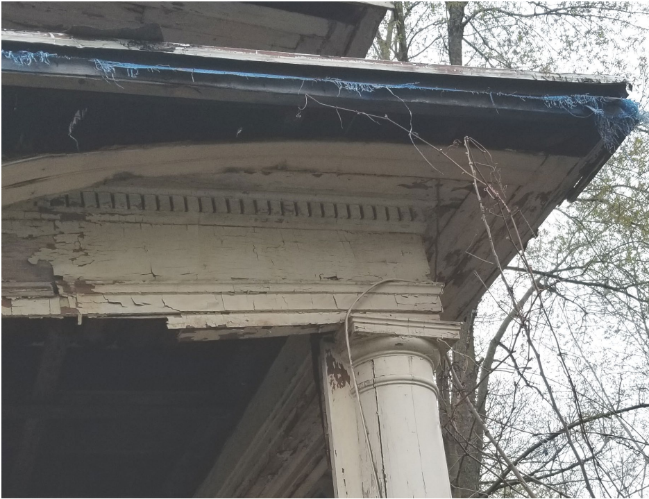
3457 Iroquois, detail, porch prior to unapproved removal
