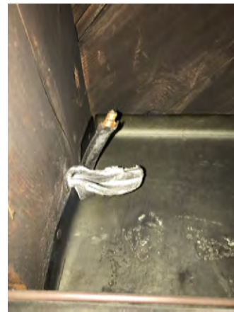
Photograph 4: Asbestos-containing woven white paper gap filler (HA21).
