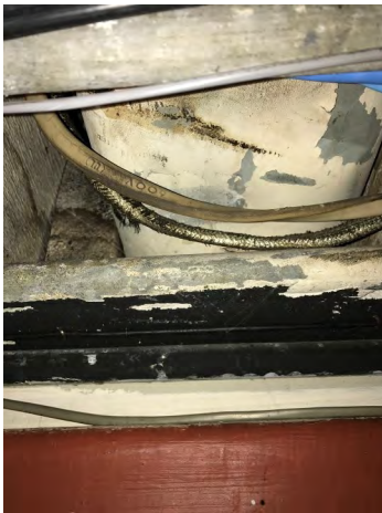
Photograph 3: Assumed asbestos-containing electrical wire wrap-white & black (HA7).
