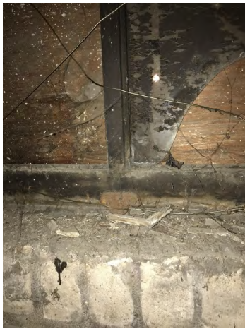
Photograph 3: Asbestos-containing white window glazing associated with basement windows (HA5).
