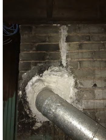
Photograph 2: Asbestos-containing mortar associated with boiler's exhaust duct (HA3).
