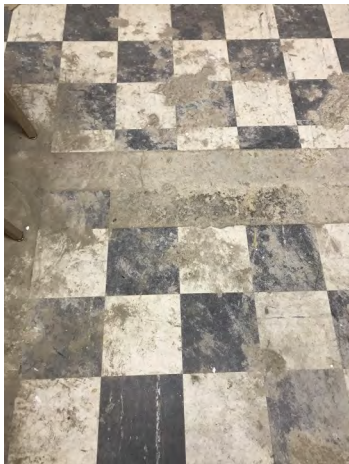
Photograph 3: Asbestos-containing 9” x 9” floor tiles-black and white intermixed (HA17). Mastics are non-ACM.
