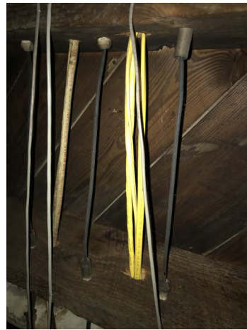
Photograph 4: Assumed asbestos-containing electrical wire wrap—white and black (HA6).
