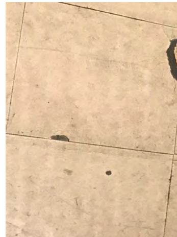
Photograph 4: Asbestos-containing 12” x 12” floor tile-light tan mottled (HA13). Mastic is non-ACM.
