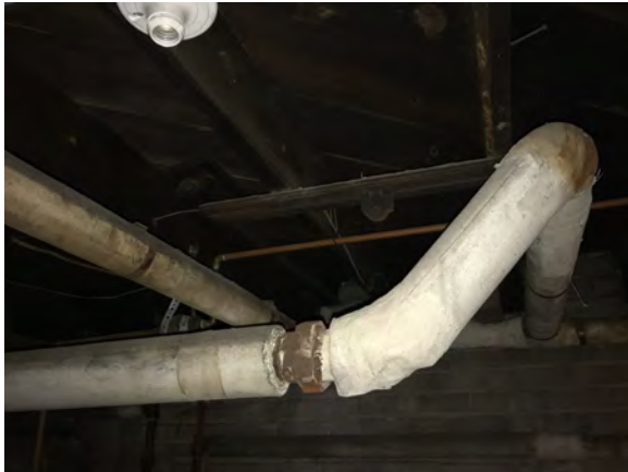
Photograph 1: Asbestos-containing aircell straight pipe insulation (HA1) and associated fitting insulation (HA2).
