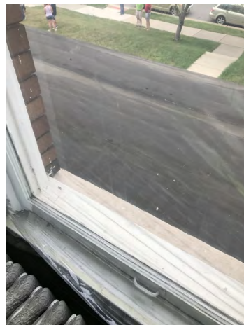
Photograph 6: Assumed asbestos-containing roofing materials above porch (HA20).
