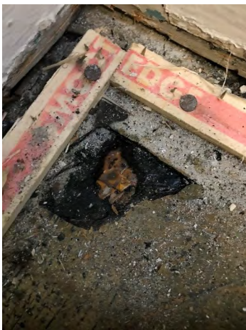
Photograph 5: Asbestos-containing 9” x 9” floor tile-black with cream streaks (HA14). Mastic is non-ACM
