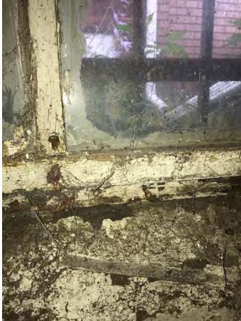
Photograph 1: Asbestos-containing window glazing associated with basement windows (H)
