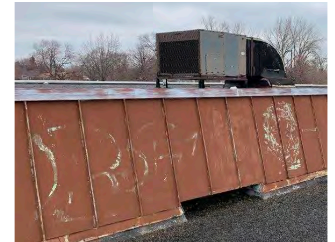
Photo R-11 / View of seamless terne standing-seam roofing with roof exhaust at sloped wall of high-bay.
