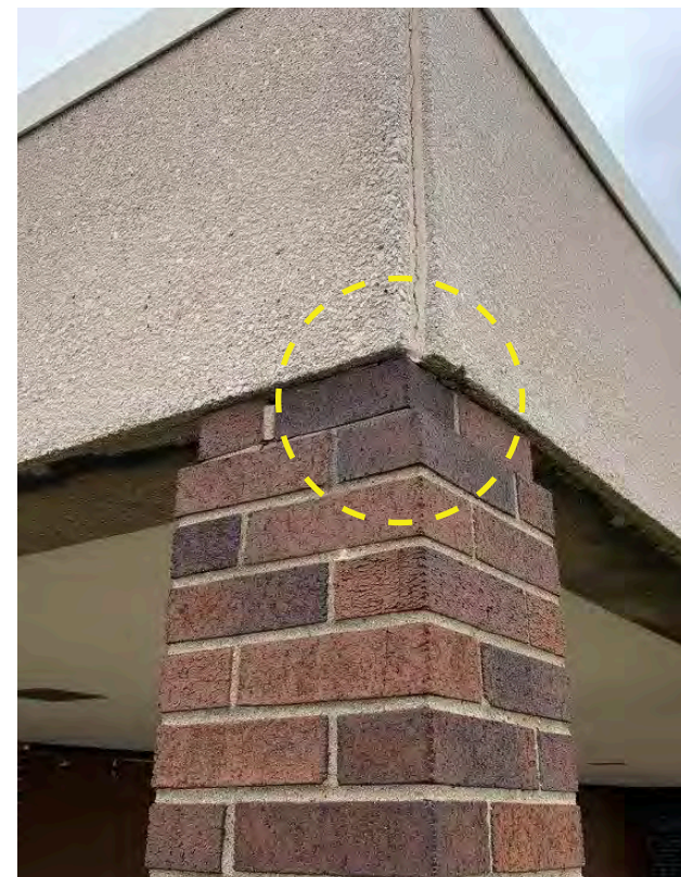
Photo S-09 / View of water damage and failing sealant in precast concrete fascia at column 4-A.
