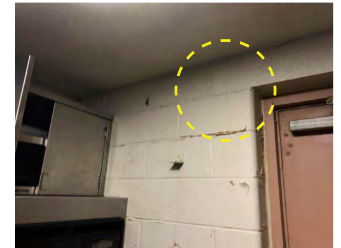
Photo I-34 / Sealant failure at perimeter of exterior door. Evidence of moisture on face of CMU walls.
