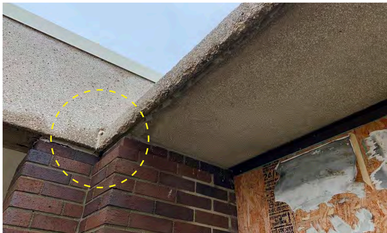
Photo S-20 / View at precast concrete canopy at B-9. Evidence of joint failure between face brick and precast concrete fascia, water damage and broken glass at window openings.
