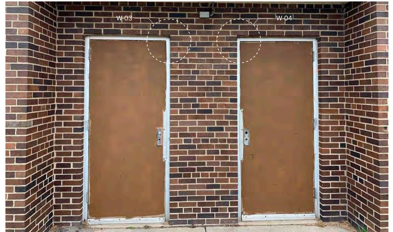
Photo W-02 / View looks SW towards exterior access to Mechanical Room (112). Door hardware is missing components. Doors are jammed in frames.
