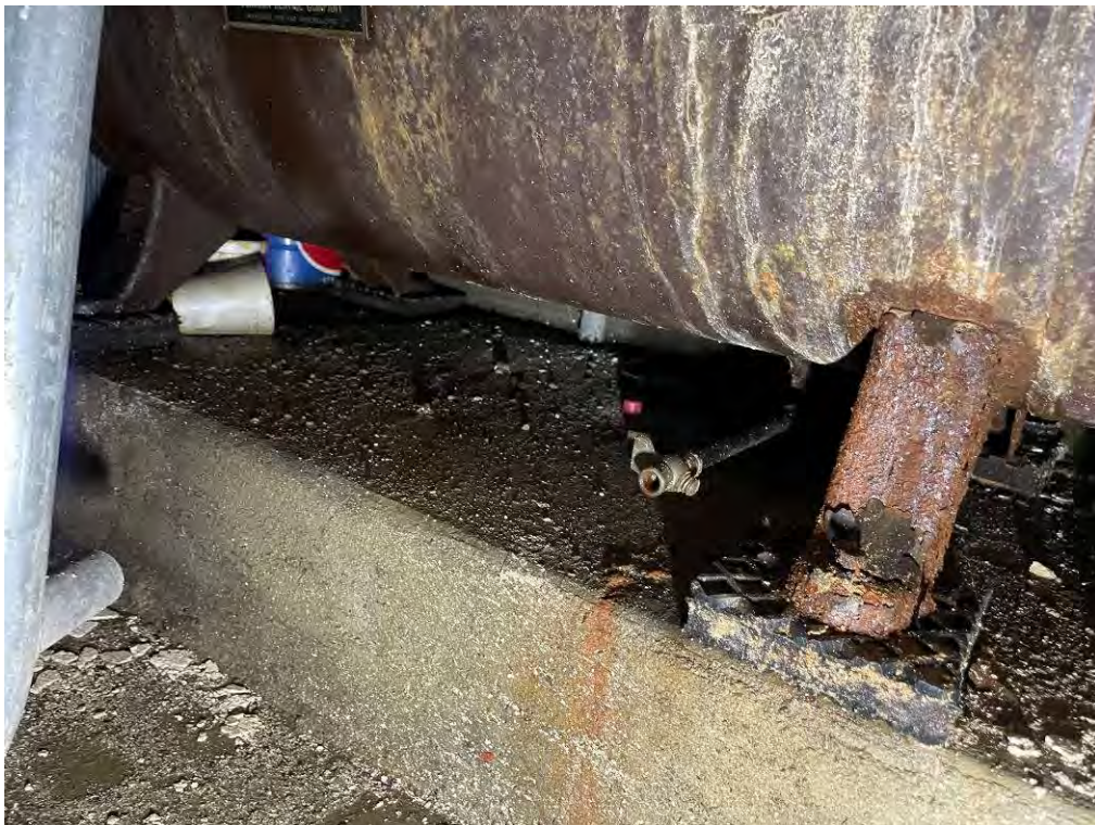
Photo 36: View of de minimis surface staining below the air compressor.
