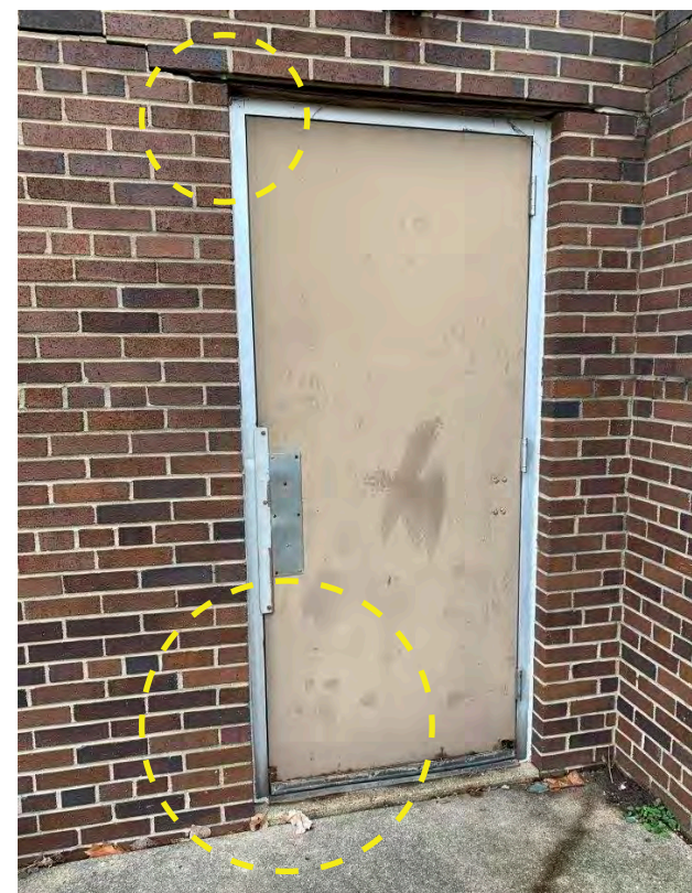
Photo N-21/ Corroded door base. Corroded steel lintels causing horizontal bed joint failure in masonry.
