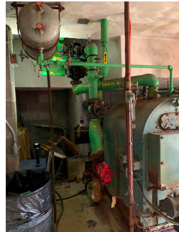
Photo M-02 / View existing boiler, expansion tank, three-way valves, pump, and associated heating hot water piping.
