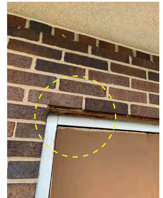
Photo W-04 / Deteriorating & corroded steel lintels causing horizontal bed joints in masonry to open.
