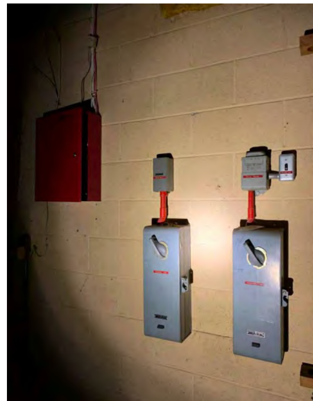
Photo I-55 / View of Storage (113) interior - Exhaust Fan controls and Security Panel on south wall.-
