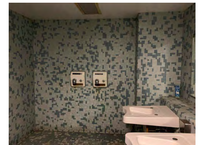
Photo I-12 / Corrosion and deterioration at wall mounted electric hand dryer.
