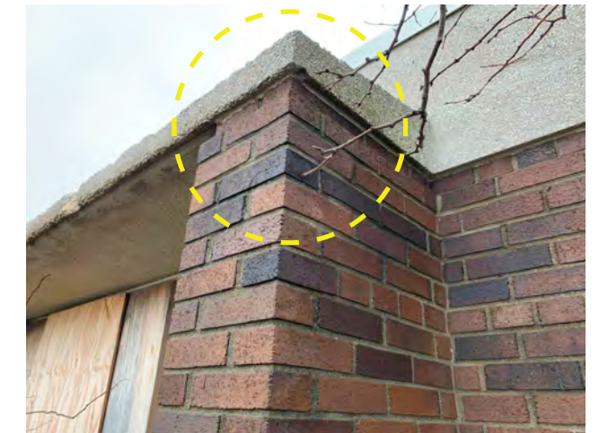
Photo S-23 / View of sealant failure and edge decay of precast concrete fascia and canopy at B-12
