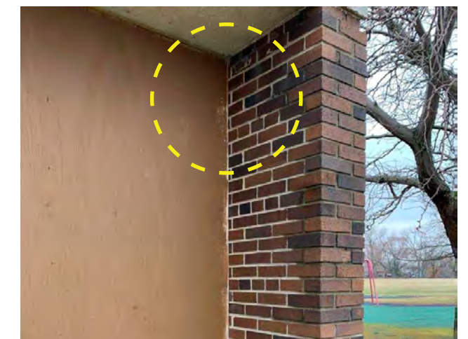
Photo S-25 / Evidence water damage and failing joints in face brick wing-wall at column B-12.
