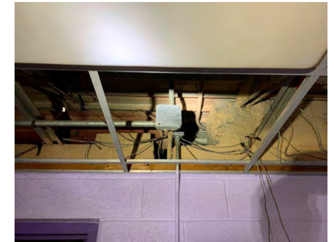
Photo I-66 / View through ceiling grid of joist framing, metal roof deck & wood nailer at perimeter.
