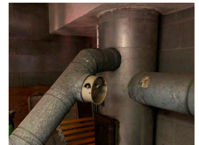
Photo M-06 / View of vents from boiler and incinerator routed through roof.
