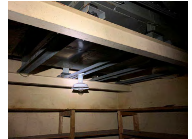
Photo I-60 / View of Heating & Ventilating Unit (HV-1) and incandescent light fixture.
