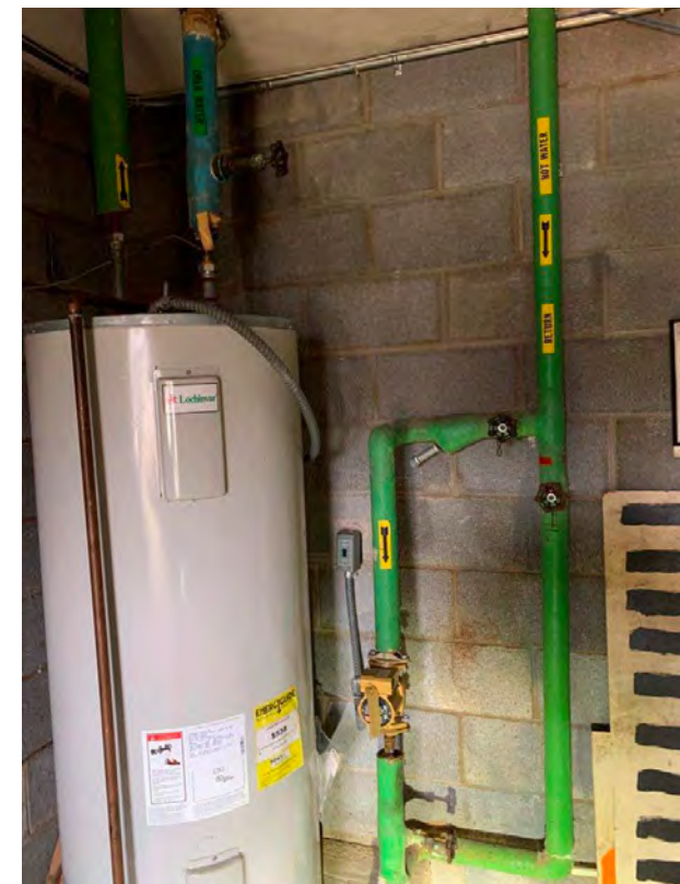
Photo M-03 / View of newer water heater and recirculation pump.
