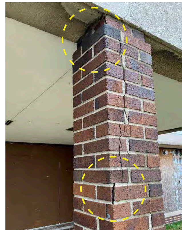
Photo S-14 / View of water damage, open joints & vertical cracking and loose brick at column 8-A.
