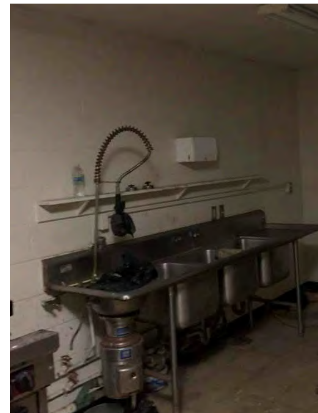
Photo I-33 / 3-compartment sink with minor corrosion and in general disrepair.
