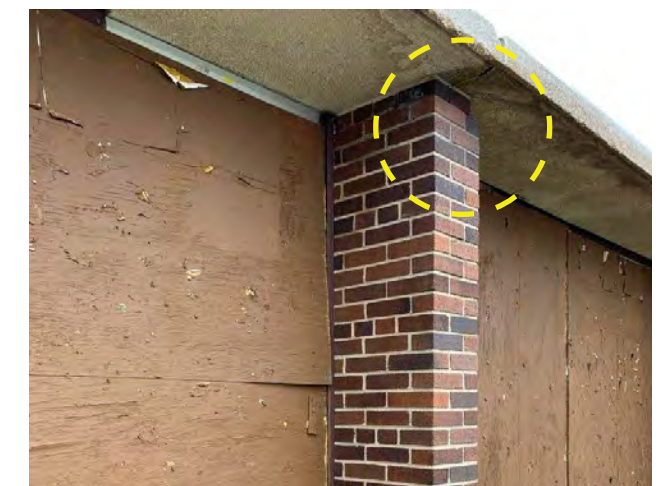
Photo S-06 / View of water damage and failure at precast concrete canopy/fascia at column B-3.
