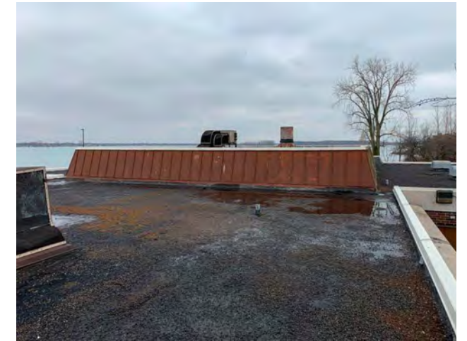
Photo R-04 / View looking West. Evidence of water ponding and aggregate loss on main roof.
