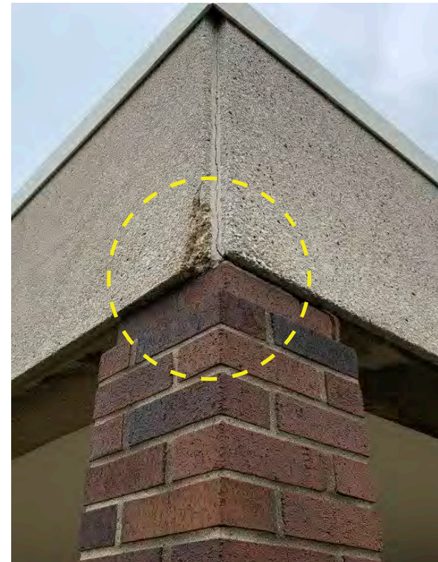
Photo S-15 / View of water damage, failing sealant and spalling precast concrete fascia at column 9-A.
