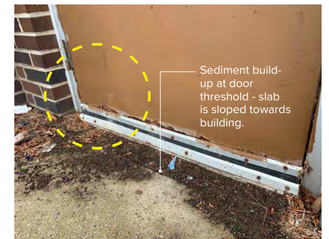
Photo E-06 / corroded door base and frame evidenced at entry.
