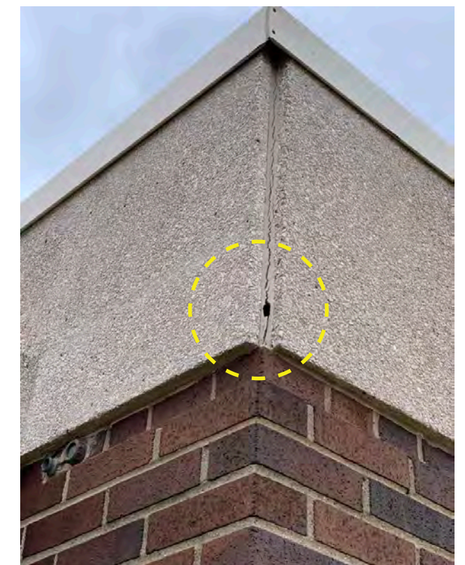
Photo N-24 / View of failing sealant in precast concrete fascia at column 1-G.
