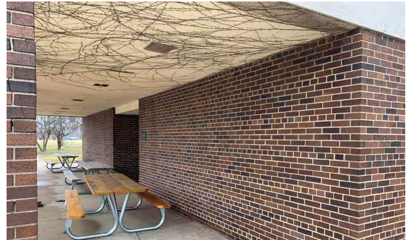
Photo N-16 / View SE towards main entrance cove. Evidence of vine growth over canopy soffit ceiling (cement plaster on metal lath) with 12" x 12" recessed incandescent light fixtures.
