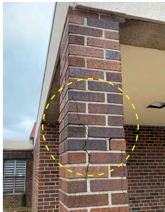
Photo N-08 / Multiple cracks through joints & brick at column 9-K. High levels of stress in the material.
