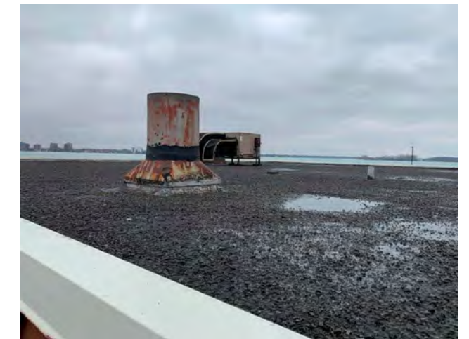
Photo R-10 / Evidence of water ponding, corroded mechanical and aggregate loss on main roof.
