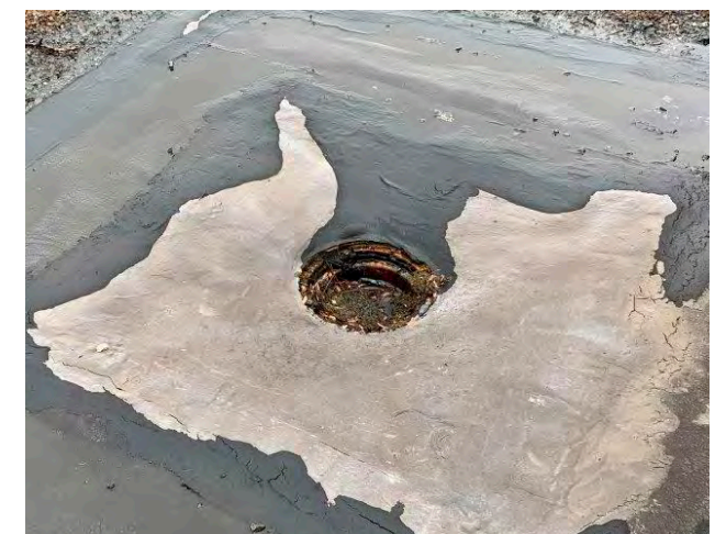
Photo R-06 / Existing roof drain (no basket strainer) and filled with debris. Drain body is corroded.
