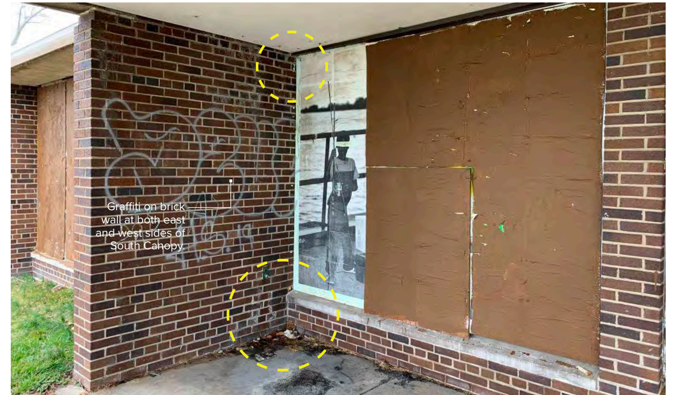
Photo S-10 / View of NW wingwall at column 4-B. Evidence of moisture damage in canopy soffit ceiling (cement plaster on metal lath). Moisture damage and efflorescence in lower brick wall. Sealant failure at window frame.
