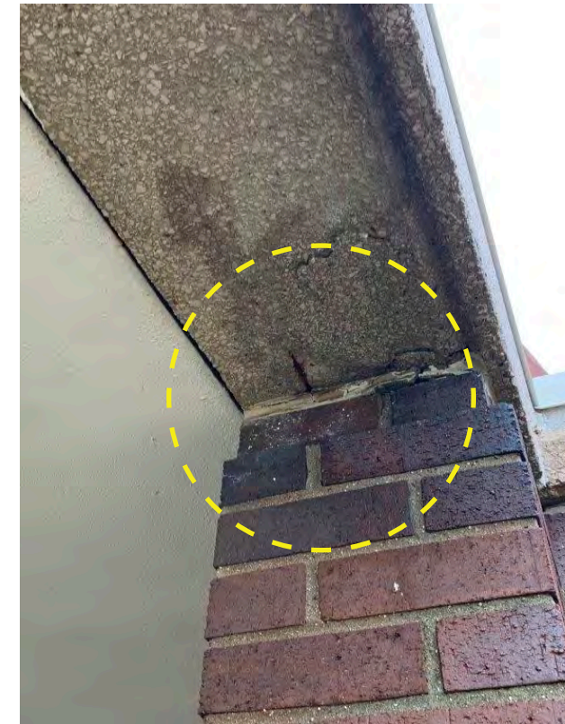
Photo S-17 / View at column-canopy joint at 9-B - joint failure, water damage & bearing plate corrosion.
