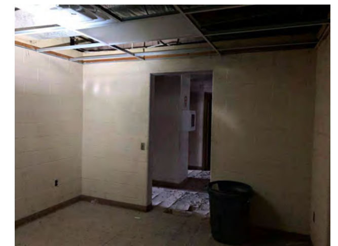
Photo I-48 / Delaminated & crumbling resilient floor tile. Corrosion evident in mechanical diffuser.
