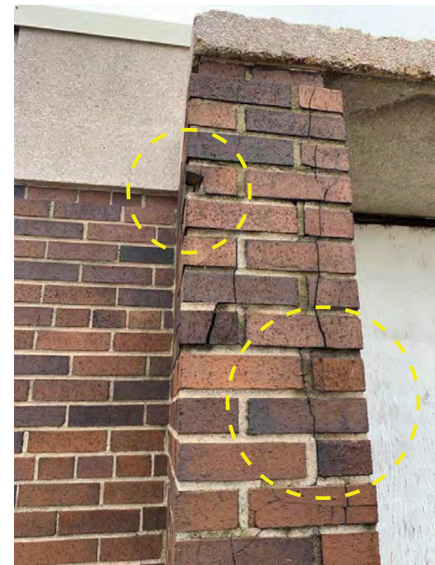
Photo S-03 / View of spalling / cracked brick and decay of precast concrete and pilaster.
