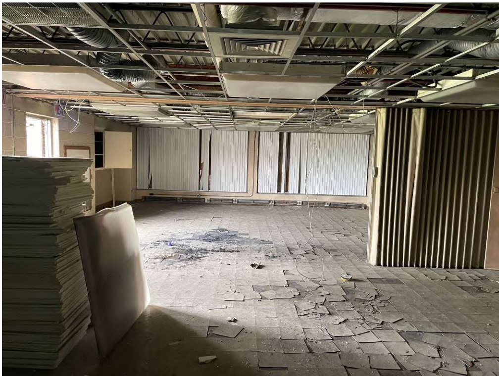
Photo 28: View of the western multi-purpose room facing north. Note the indications of a fire on the floor.
