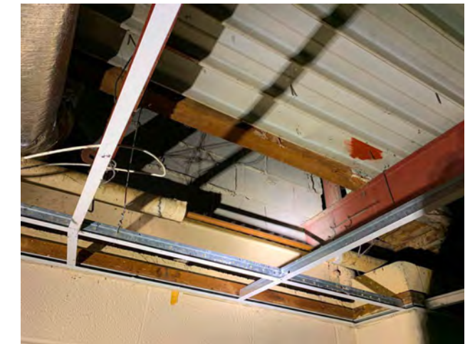
Photo I-46 / View through ceiling grid of insulated piping, duct work and metal roof deck.
