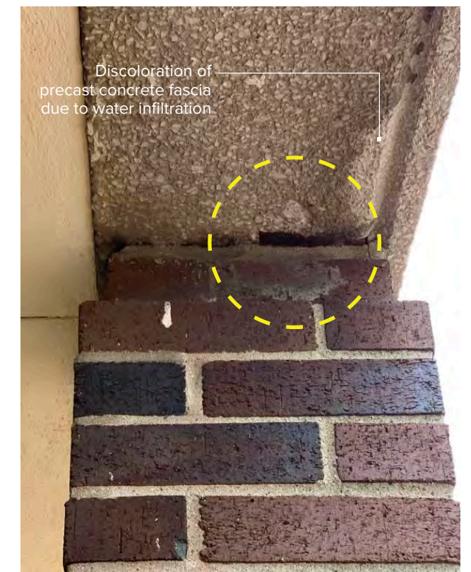
Photo N-18 / View at column-canopy joint at 5-K - joint failure and evidence of bearing plate corrosion.
