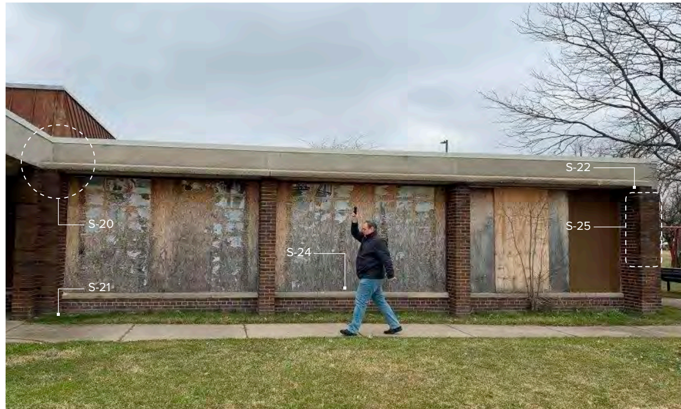
Photo S-19 / Partial view of South Elevation / East Wing. Protective plywood sheathing has been fastened through aluminum storefront framing. Glass behind is shattered or missing.
