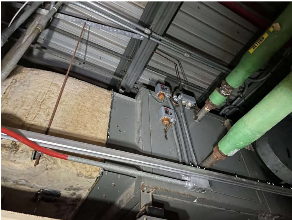
Photo 20: View of interior mounted HVAC equipment within the eastern storage HVAC room.
