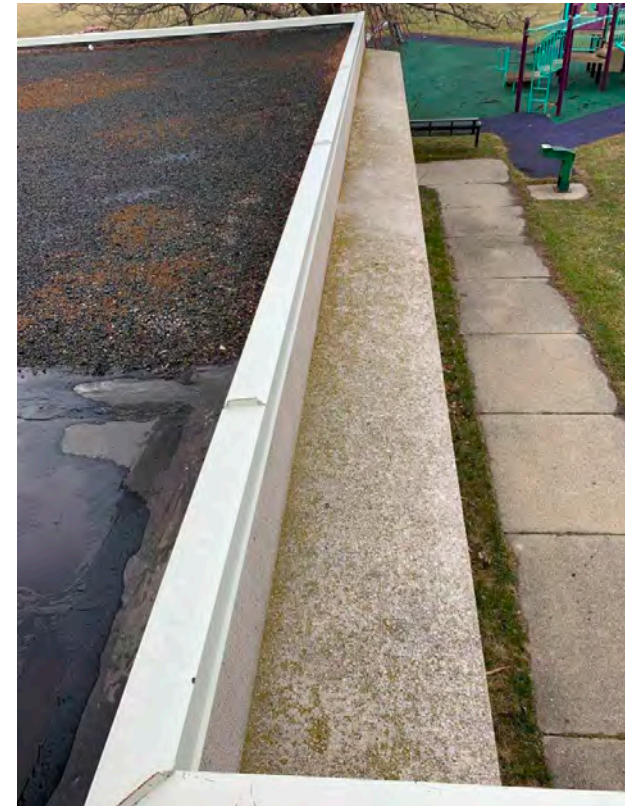
Photo R-02 / View of cap flashing over precast concrete fascia & canopy with pitting evident
