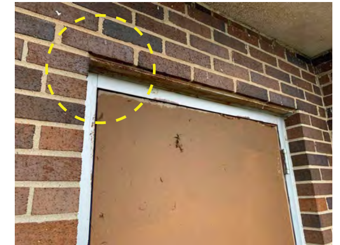
Photo E-05 / Evidence of corroded steel lintel and open joint in masonry above door opening.
