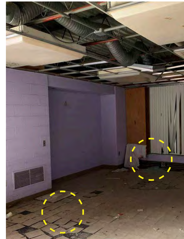
Photo I-63 / Covers removed and heavy corrosion in electric base board radiators. Ceiling tiles removed.
