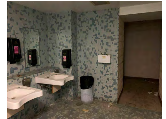
Photo I-11 / Wall-mounted lavatory and pipe protection panel is non-compliant with ADA regulations.
