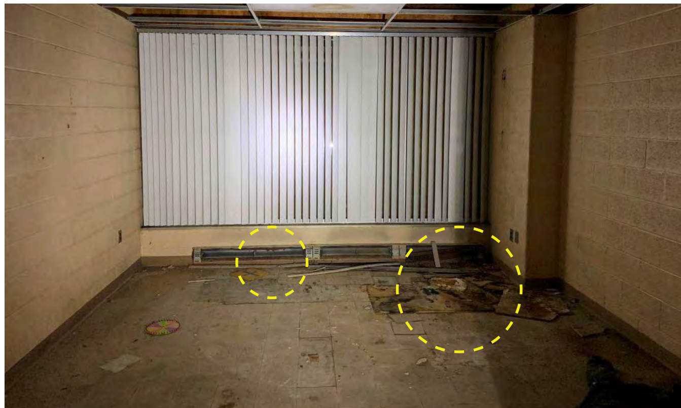
Photo I-68 / Overall view of Reading Room (110). Aluminum window frames have been compromised by fastening of plywood sheathing. Glazing has been removed. Electric base board radiators have been damaged and are corroding.
