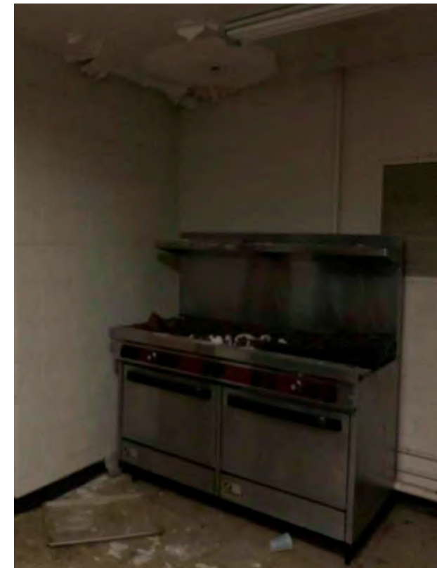
Photo I-32 / Range/oven with minor corrosion and in general disrepair. Moisture damage evident at plaster ceiling. Resilient tile broken & delaminating from slab..
