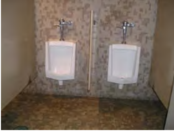
Picture left shows the urinals in the men's restroom. The partitions are rusting.
