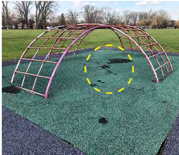
Photo ST-18 / View of corroded play structure.
