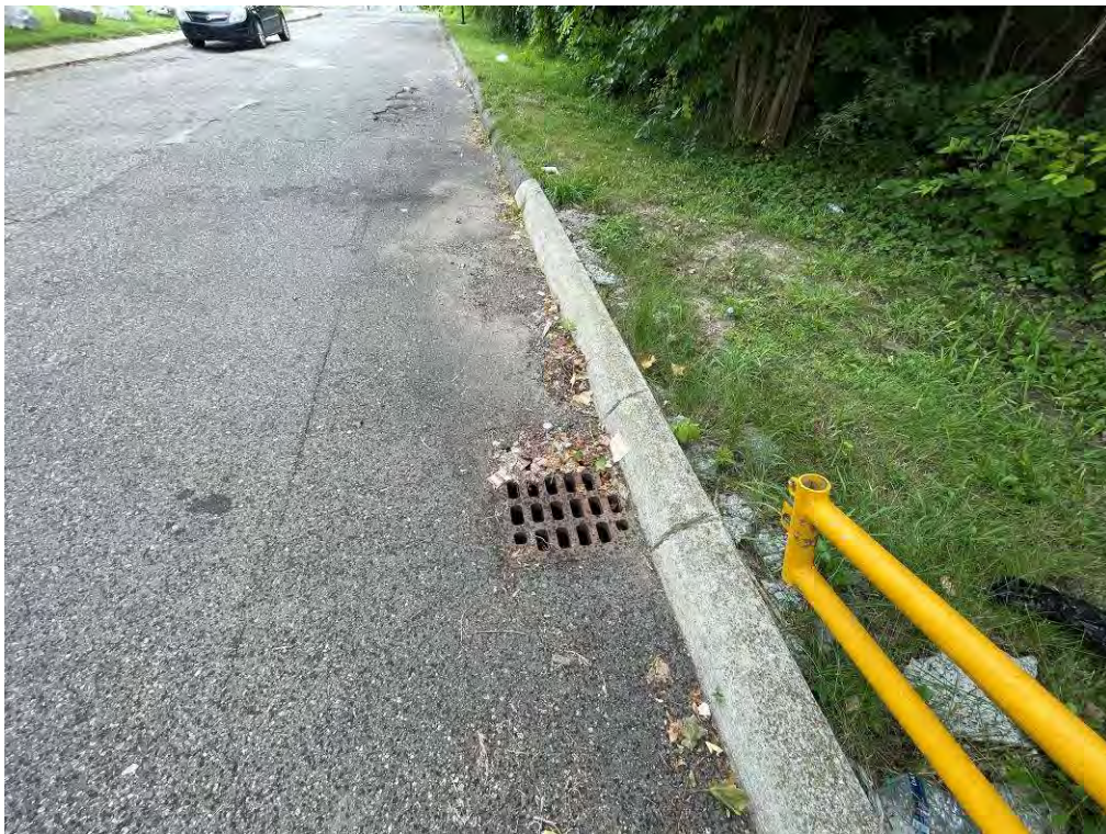
Photo 46: View of a typical stormwater catch basin.
