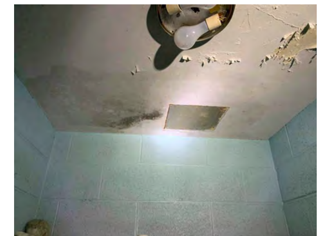
Photo I-61 / Delaminated & crumbling plaster ceiling with evidence of mold. Corrosion fixture housing.
