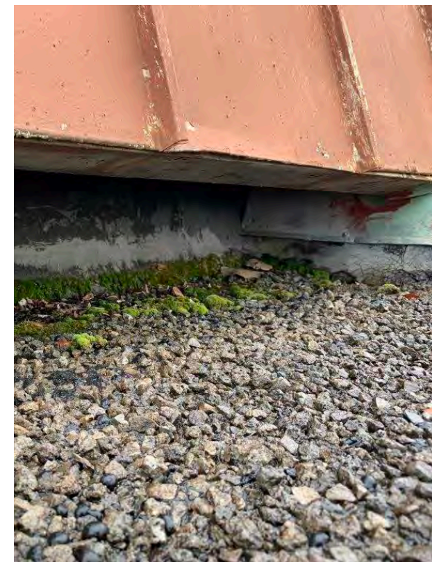
Photo R-09 / Evidence of sealant failure, sheathing decay at roof exhaust & cracking at BUR.
