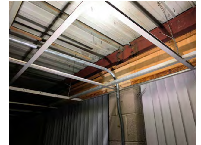
Photo I-41 / View through ceiling grid of steel beam framing, metal roof deck & plywood cove at perimeter.
