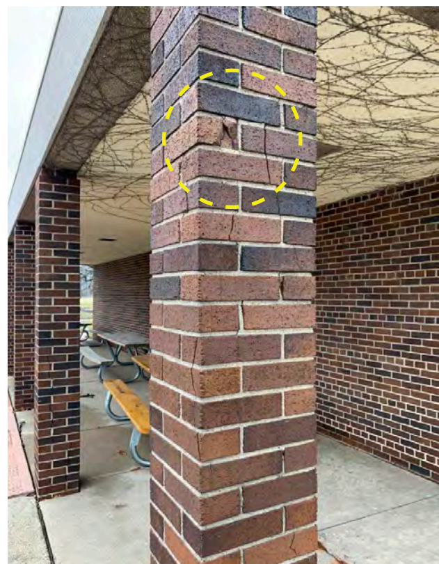
Photo N-14 / Multiple cracks through joints & brick at column 4-K. High levels of stress in the material.
