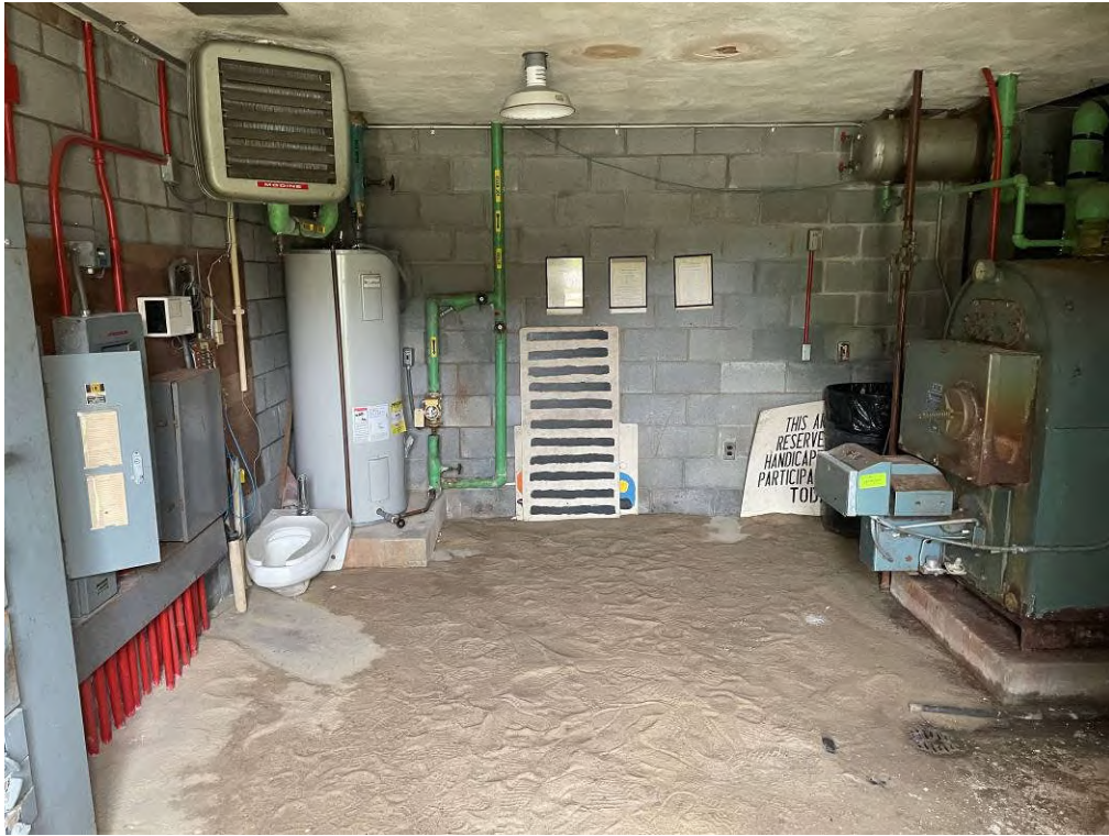
Photo 31: View of the eastern mechanical room. Note the silt on the floor indicative of water intrusion.
