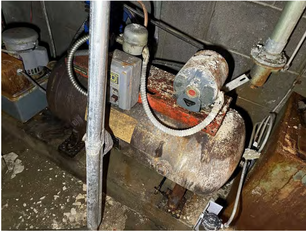
Photo 35: View of air compressor located within the mechanical room.
