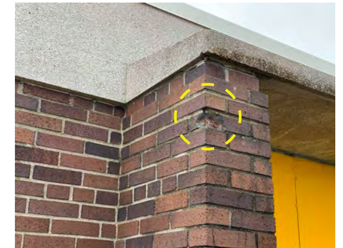
Photo N-04 / View of spalling face brick and sealant failure at precast concrete fascia and canopy.
