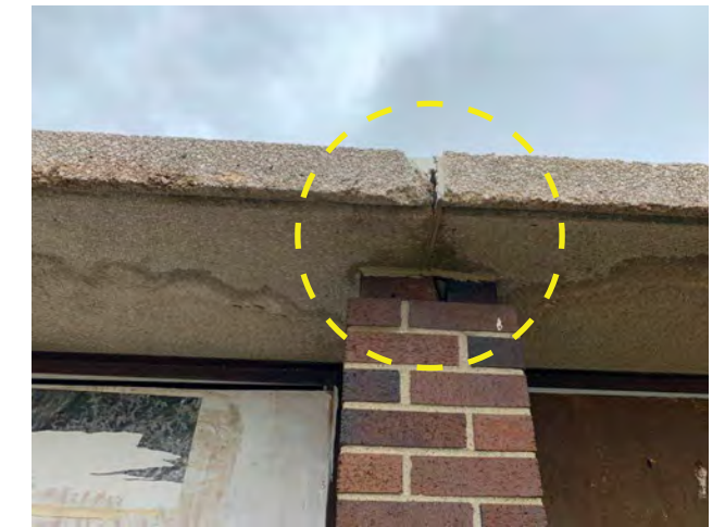
Photo S-04 / View of water damage and failure at precast concrete canopy/fascia at column B-2.
