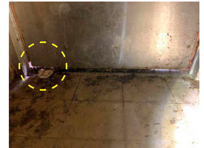
Photo I-22 / Corroded door base and threshold in Women's Coat Room (103)
