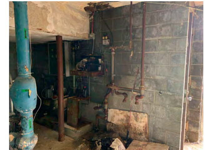
Photo M-05 / View of where existing gas meters were located. Meters have been removed.
