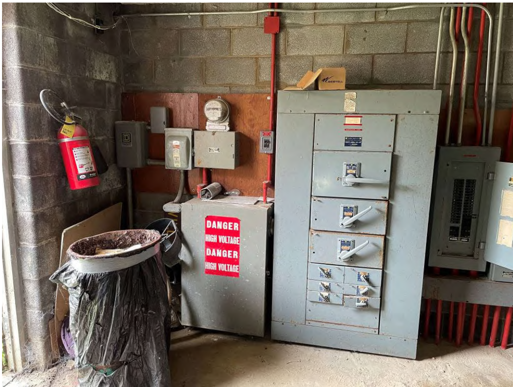
Photo 32: View of electrical equipment and 35-gallon salt drum located within the mechanical room.
