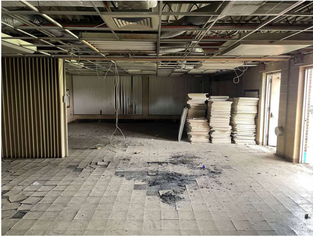
Photo 27: View of the western multi-purpose room facing south. Note the indications of a fire on the floor.
