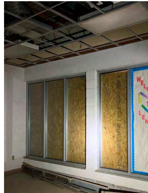
Photo I-50 / Covers removed and heavy corrosion in electric base board radiators. Ceiling tiles removed. Glazing damaged or missing in some frames.
