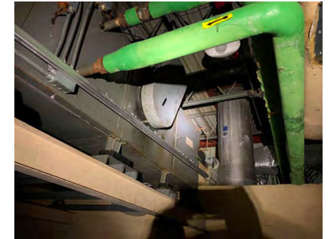
Photo I-59 / Storage (113) - View of Heating & Ventilating Unit (HV-1)
