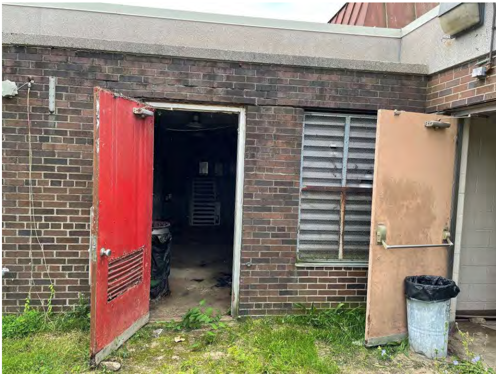
Photo 30: View of the eastern mechanical room via the exterior entrance.
