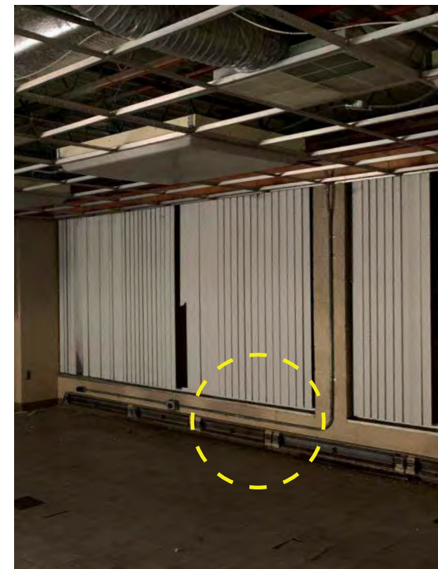
Photo I-39 / Covers missing & corrosion in electric base board radiators. Window blinds in poor condition.
