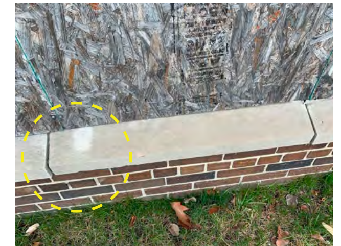
Photo S-24 / Evidence of broken glazing and loss of joint material between precast concrete sill.
