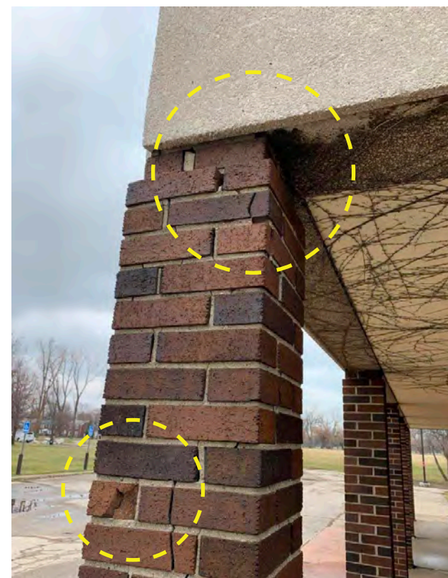
Photo N-15 / Multiple cracks through joints & brick at column 4-K. High levels of stress in the material.
