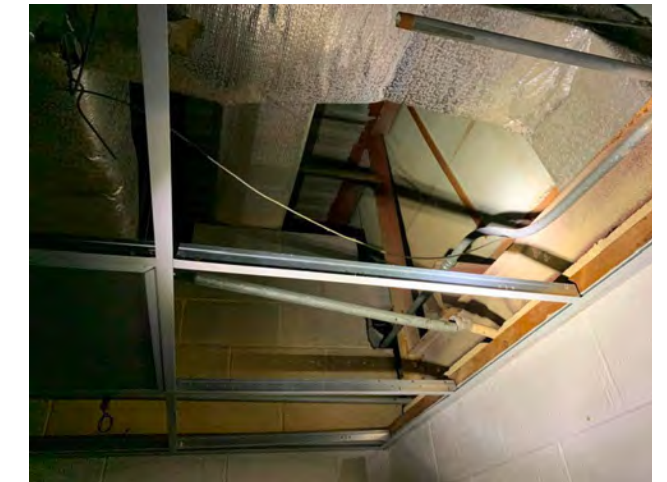
Photo I-29 / View through ceiling grid of insulated ducts, steel joist framing and metal roof deck.
