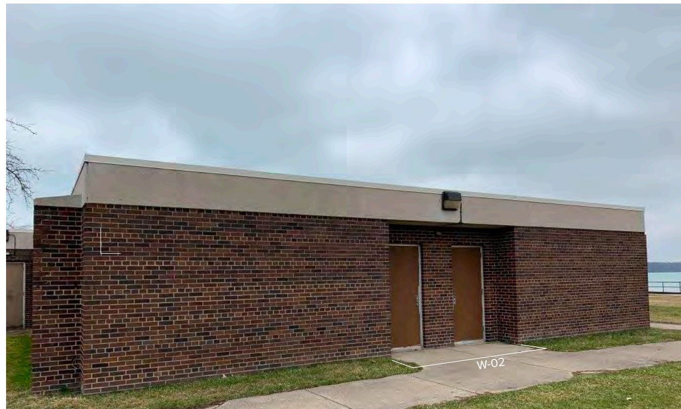
Photo W-01 / Overall view of West Elevation. Face brick is in Good to Fair position on this side of the building.
