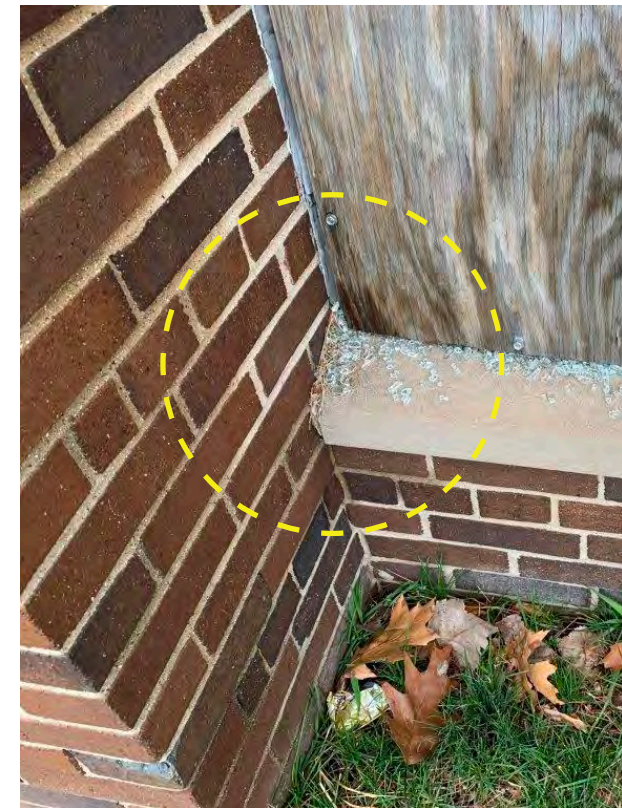
Photo S-21 / Broken glazing and plywood has been fastened through aluminum window frame.
