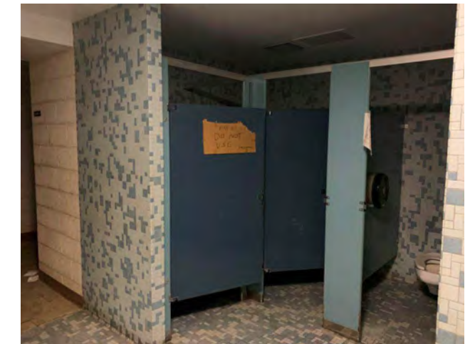
Photo I-10 / View of floor mounted partitions with signs of delaminating finish, corrosion & deterioration.
