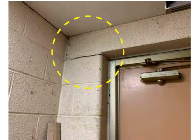
Photo I-23 / Failure in joint at concrete door lintel and translated cracking along CMU wall and plaster ceiling.
