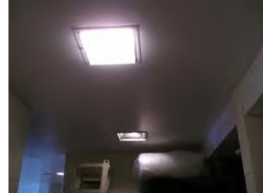
Picture right shows a ceiling in the hallway near the men's restroom. One of the light fixture covers is missing.
