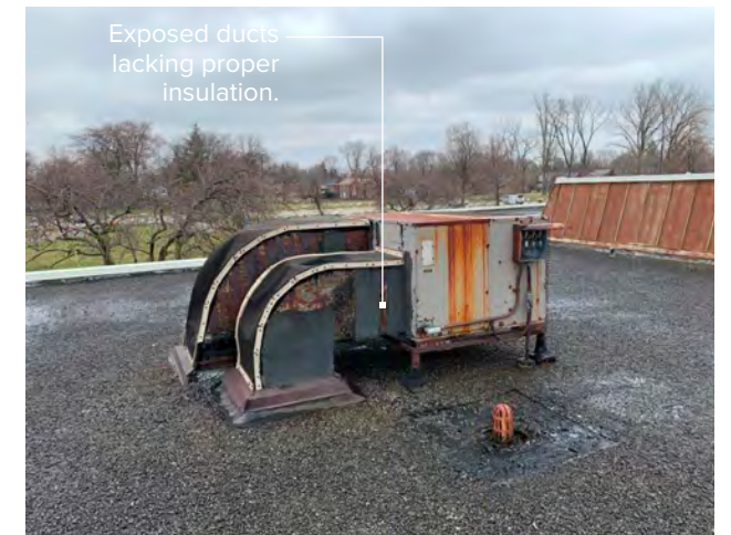
Photo R-05 / Existing air cooled rooftop air conditioner with supply & return ductwork through the roof.
