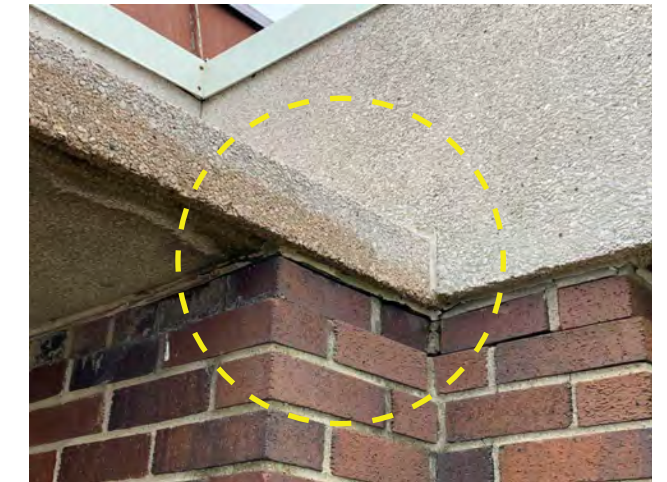
Photo S-05 / View of cracked face brick and sealant failure at precast concrete fascia and canopy.
