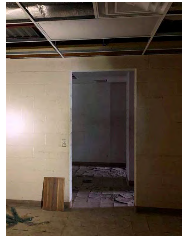
Photo I-70 / Delaminated & crumbling resilient floor tile.
