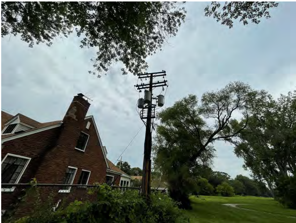
Photo 12: View of three pole-mounted electrical transformers located along the northern subject property boundary.
