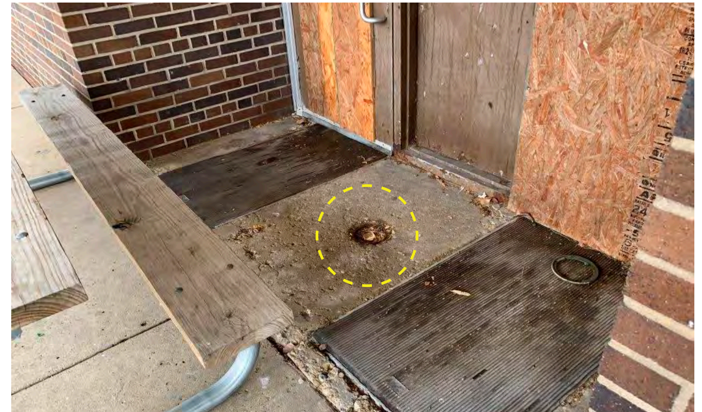
Photo N-10 / View of main entrance in north elevation. Existing clean-out for main sanitary line is corroded and filled with debris. Evidence of heaving, deteriorating and pitted concrete slab. Recessed entrance mats at both doors are corroded and decaying. Hollow metal doors and frame in Fair to Poor condition.
