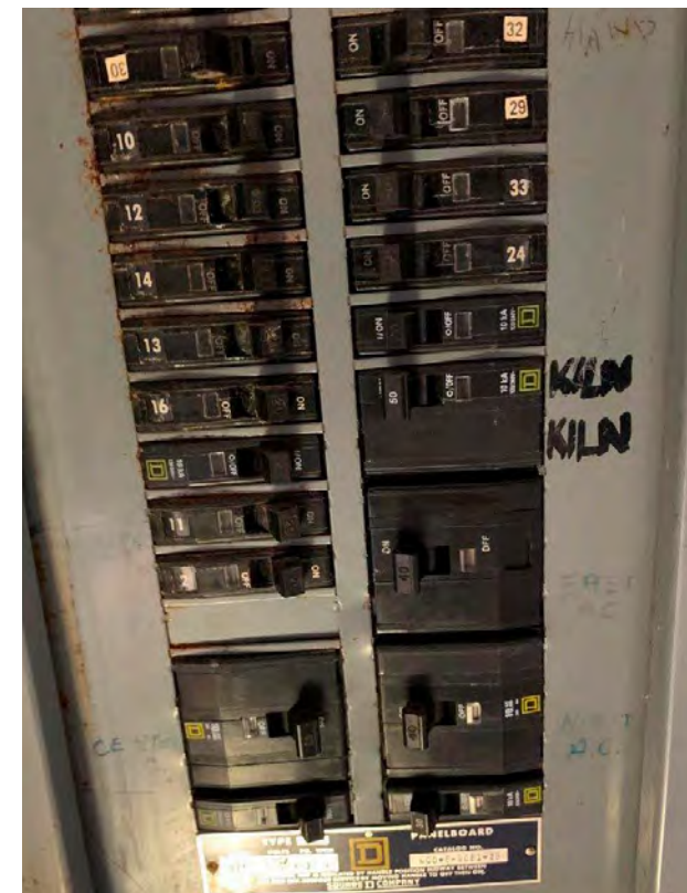
Photo E-04 / View of existing Square D Panel.
