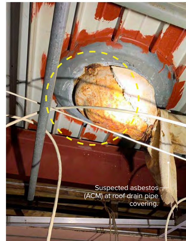
Photo I-64 / Failing roof sump. Water has infiltrated the interior of Multi-Purpose Room.
