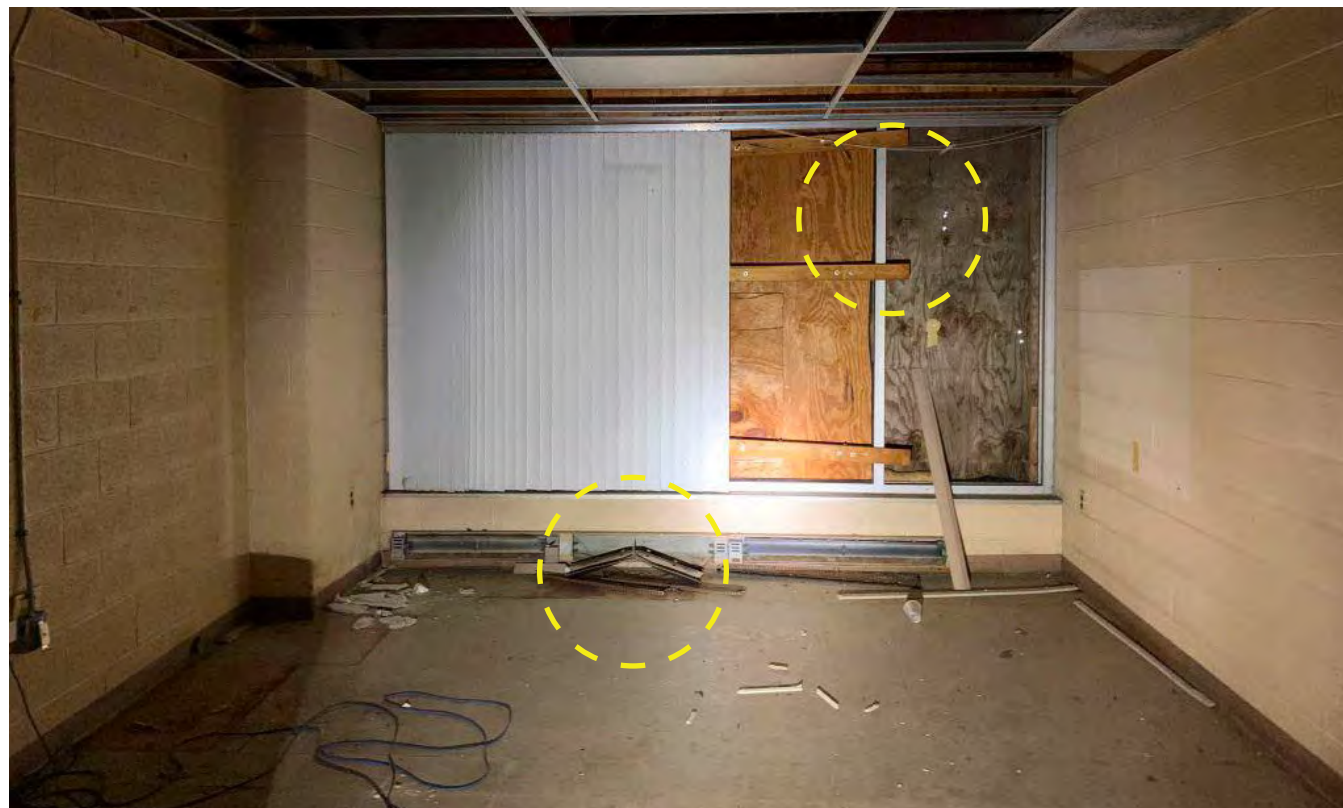
Photo I-43 / Overall view of Games Room (108). Aluminum window frames have been compromised by fastening of plywood sheathing. Glazing has been removed. Electric base board radiators have been damaged and corroding.
