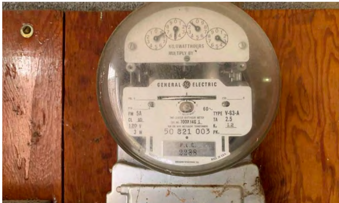
Photo E-02 / View of wall mounted meter in Mechanical Room (112).
