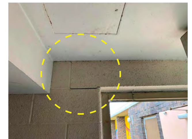
Photo I-24 / Failure in joint at concrete door lintel.
