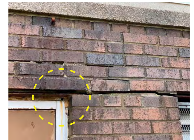
Photo N-05 / Deteriorating & corroded steel lintels causing horizontal bed joints in masonry to open.
