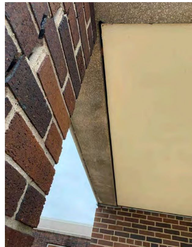
Photo N-09 / View of north canopy ceiling (cement plaster on metal lath) with precast concrete fascia.
