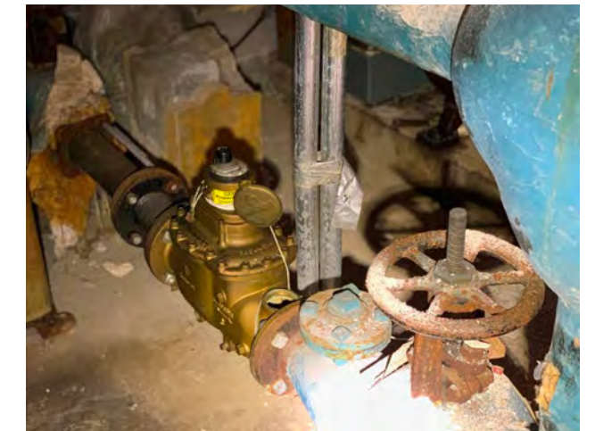
Photo M-04 / View of existing 3" water meter with unknown water service pipe size.
