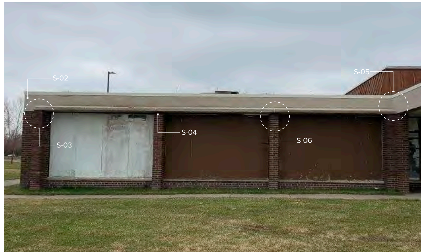
Photo S-01 / Partial view of South Elevation / West Wing. Protective plywood sheathing has been fastened through aluminum storefront framing. Glass behind is shattered or missing.
