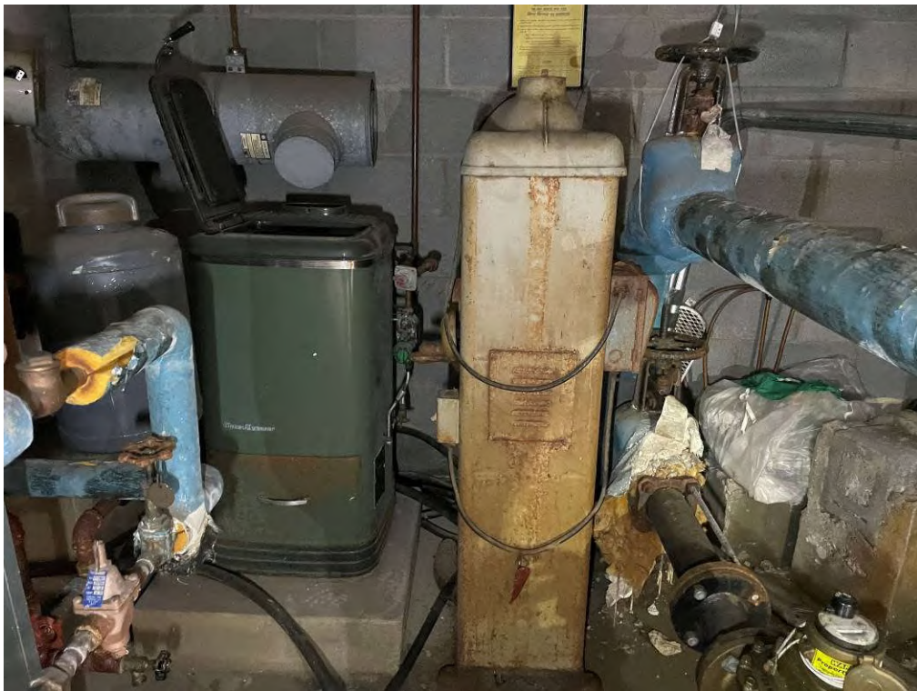
Photo 34: View of incinerators located within the mechanical room.
