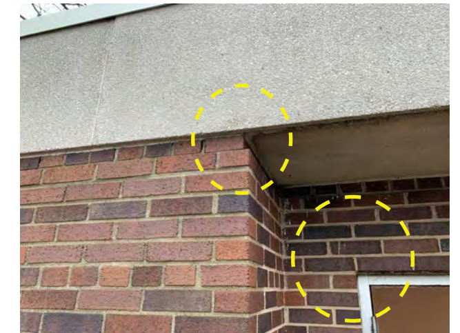
Photo E-04 / Sealant failure in joint between precast concrete fascia and soffit.
