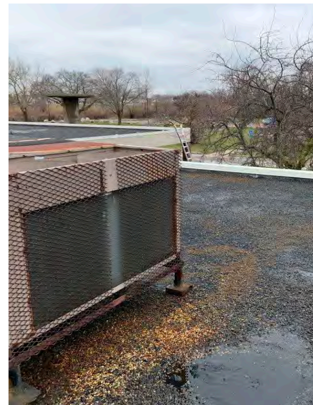
Photo R-03 / Evidence of ponding water and aggregate loss at Built-Up Roof. Corroded Mech. Unit.
