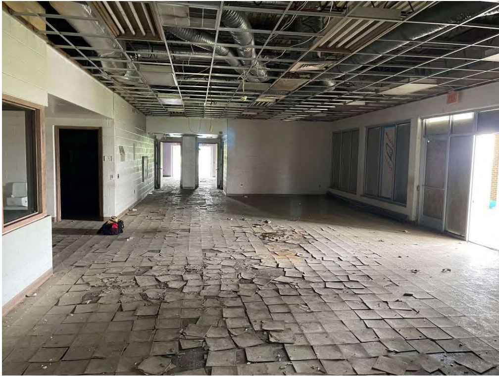
Photo 23: View of the large lounge. Note a 2013 water main break caused extensive damage and the building was permanently closed.
