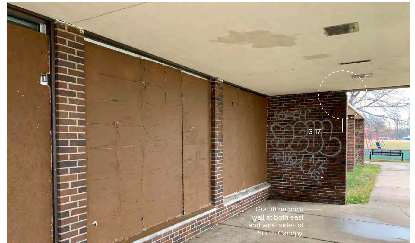
Photo S-16 / View of NE wingwall at column 9-B. Evidence of moisture damage in canopy soffit ceiling (cement plaster on metal lath). Moisture damage brick wall wing-wall. Sealant failure at window frame with broken glass.
