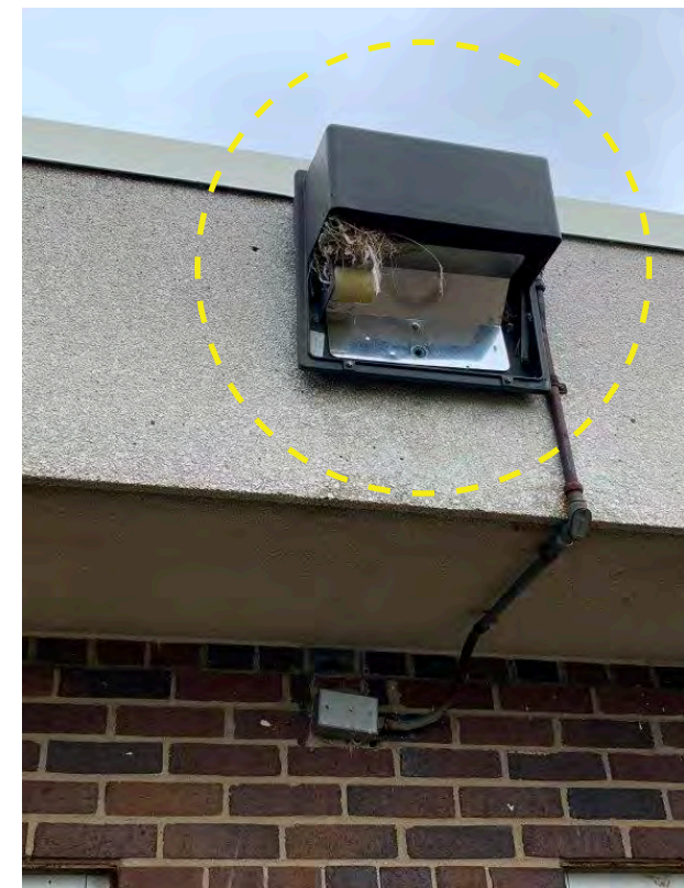
Photo E-03 / Damaged surface mounted light fixture.
