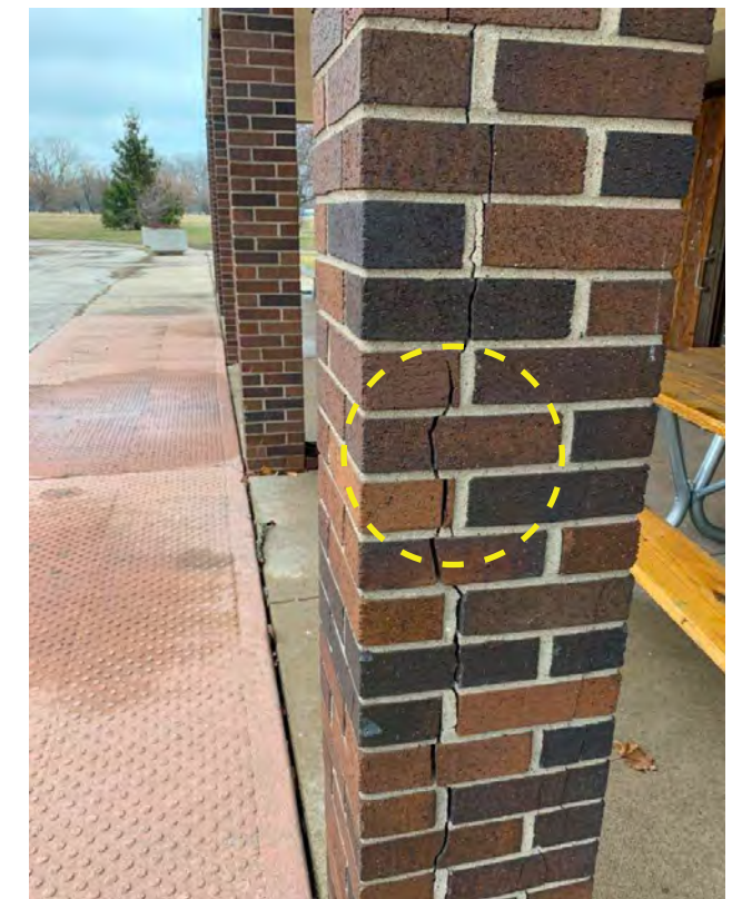
Photo N-12 / Full length crack through joints & brick at column 5-K. High levels of stress in the material.
