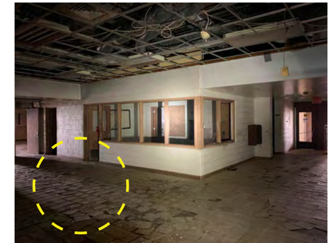
Photo I-52 / View towards Office (105). Delaminated & crumbling resilient floor tile. Ceiling Tile removed.
