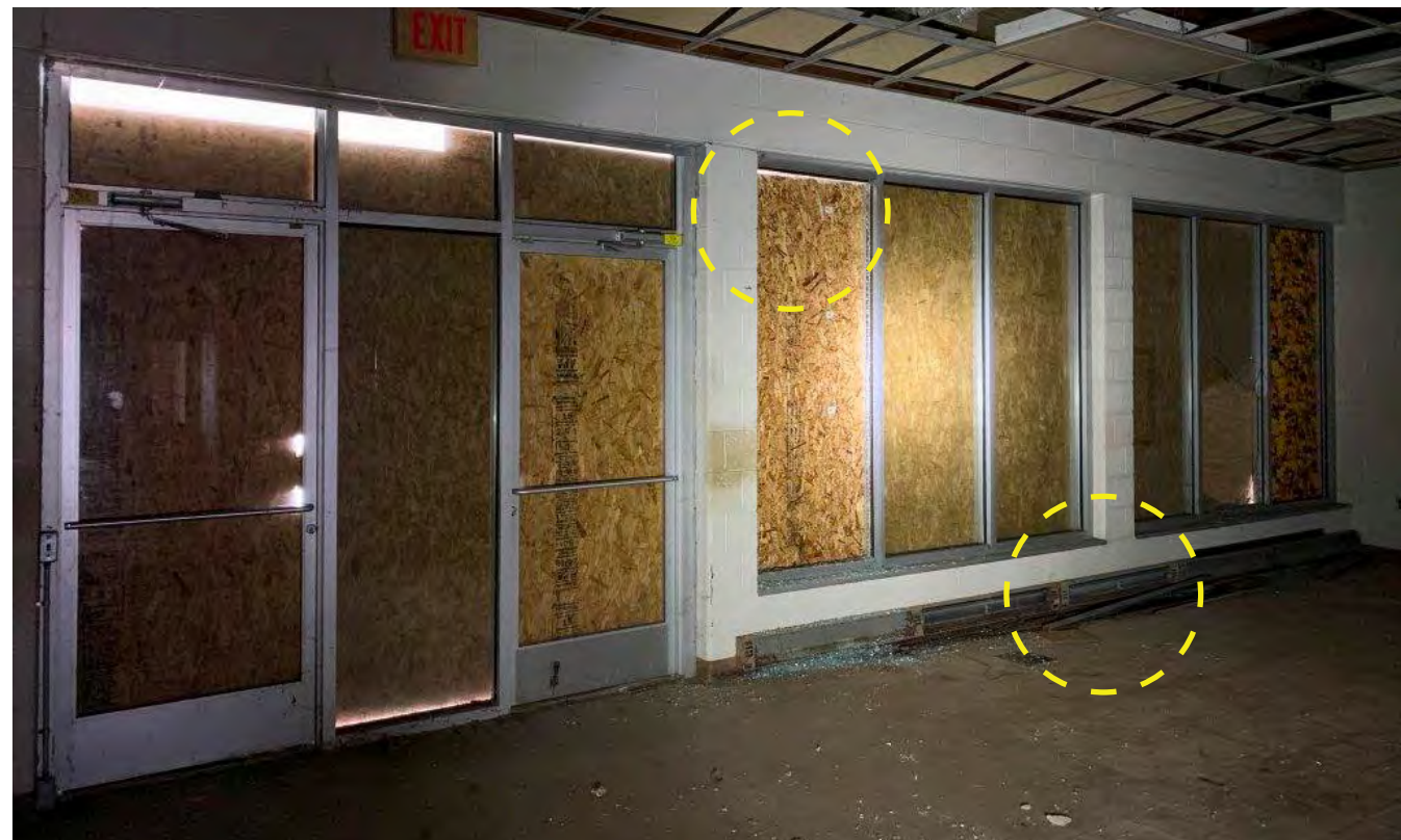
Photo I-49 / Aluminum window frames have been compromised by fastening of plywood sheathing. Glazing has been vandalized in several locations. Electric base board radiators have been damaged and are heavily corroded.
