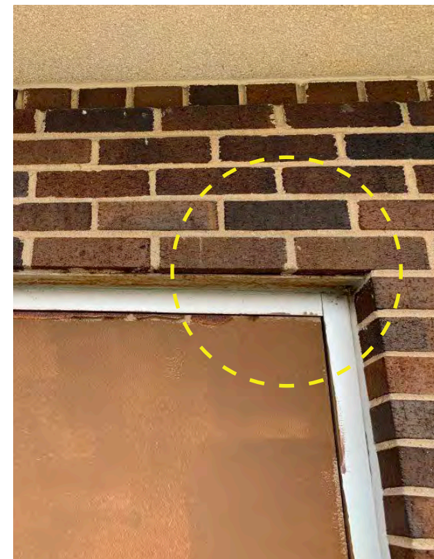
Photo W-03 / Minor corrosion in steel lintels and door leaf. Door hardware absent.
