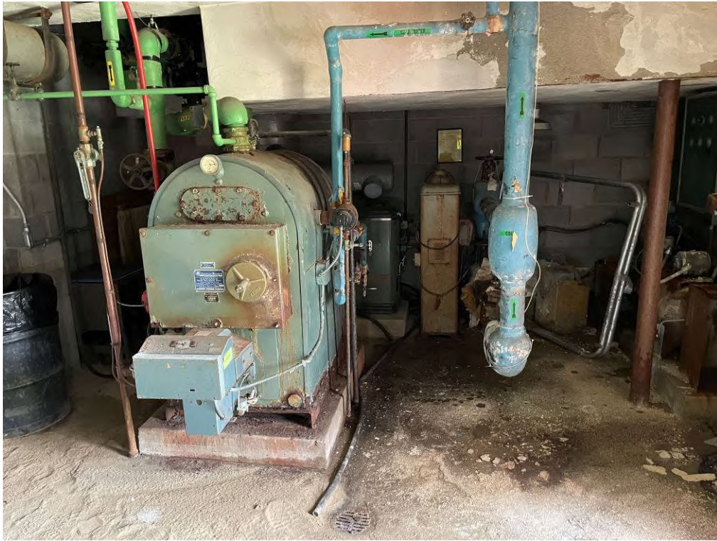
Photo 33: View of electrical equipment and 55-gallon general refuse drum located within the mechanical room.
