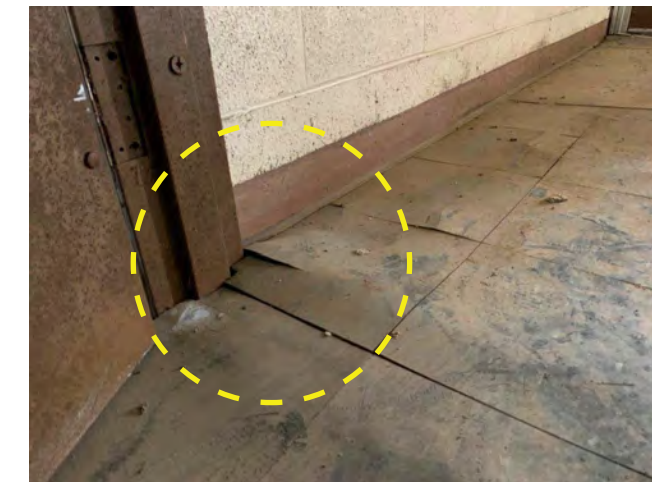
Photo I-05 / View of corroded frame, water damaged and delaminating resilient tile at Vestibule floor.
