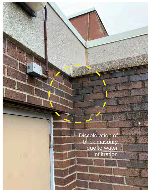
Photo N-20 / Joint openings allow water ingress which will has exacerbated freeze-thaw deterioration.
