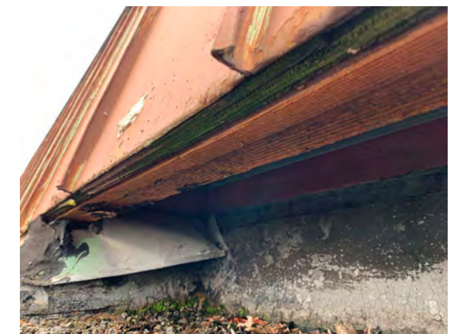
Photo R-12 / Evidence of sealant failure at flashing, moisture damage to wood & cracking at BUR.
