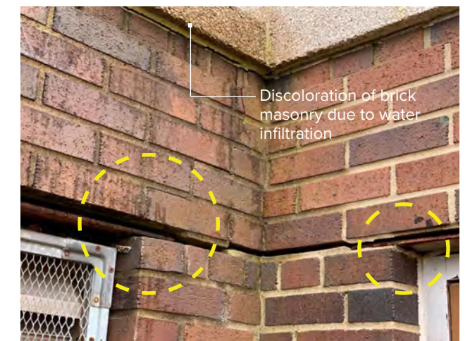
Photo N-06 / Deteriorating & corroded steel lintels causing horizontal bed joints in masonry to open.
