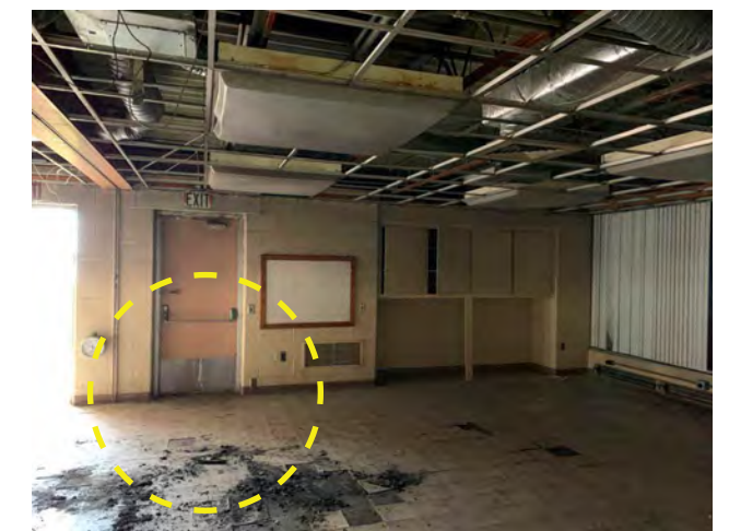
Photo I-42 / Delaminated & crumbling resilient floor tile. Corrosion evidenced in light fixture housing.
