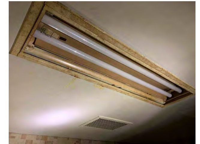
Photo I-17 / View of corroded recessed 1x4 fluorescent troffer in plaster ceiling.
