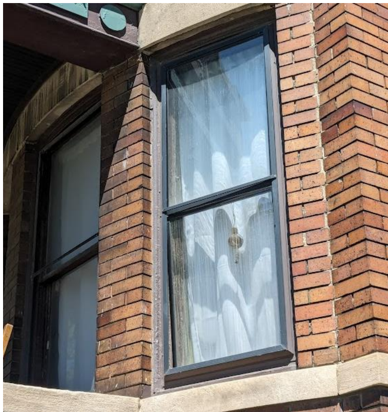
Existing condition showing historic sash window, wood brickmould trim, and storm window track fastened to brickmould. Note: photo is of the 1028 Vinewood half of the building due to greater visibility, but the condition is the same. May 2024 Photo by staff.
