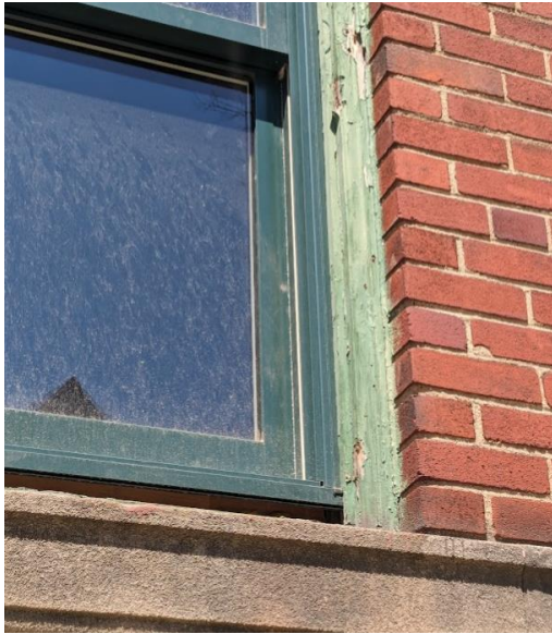
Example (from another property) of a window installed within a sash box, reducing the size of the opening. This is an inappropriate installation. May 2023 photo by staff.
