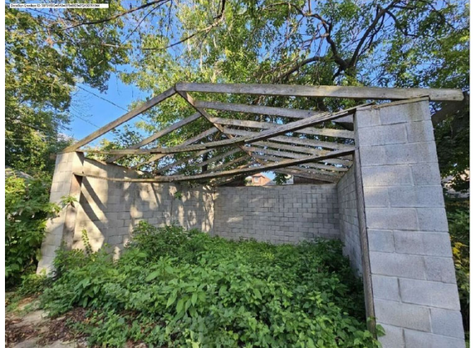
Site Photo 2, by Applicant: (Looking east at rear of property) showing partially constructed garage structure (without approval).
