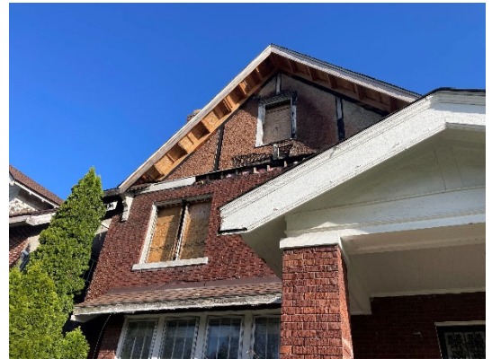
Site Photo 4, by Staff April 19, 2024: (South) front elevation showing detail of missing windows, soffit, stucco and half-timbering.
