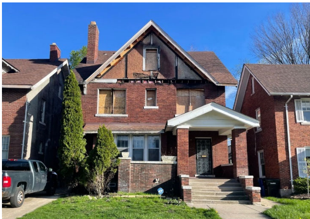
Site Photo 1, by Staff April 19, 2024: (South) front elevation showing fire damage at front gable and missing windows.
