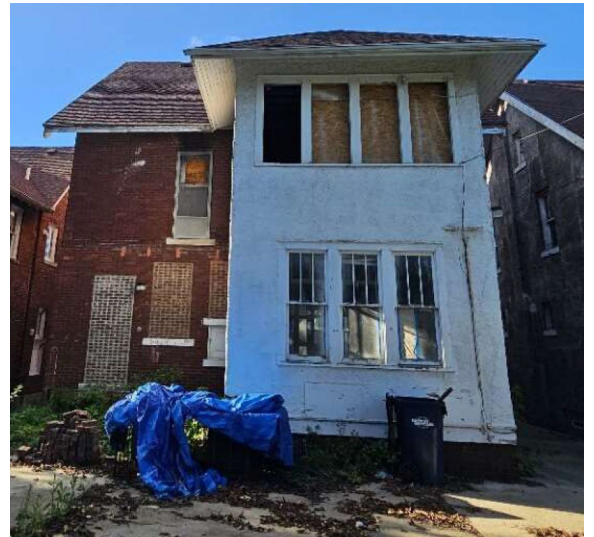
Site Photo 3, by Applicant: looking north (rear) side of the house, showing unapproved removal of balcony/porch, bricked-in openings of the rear door and windows.
